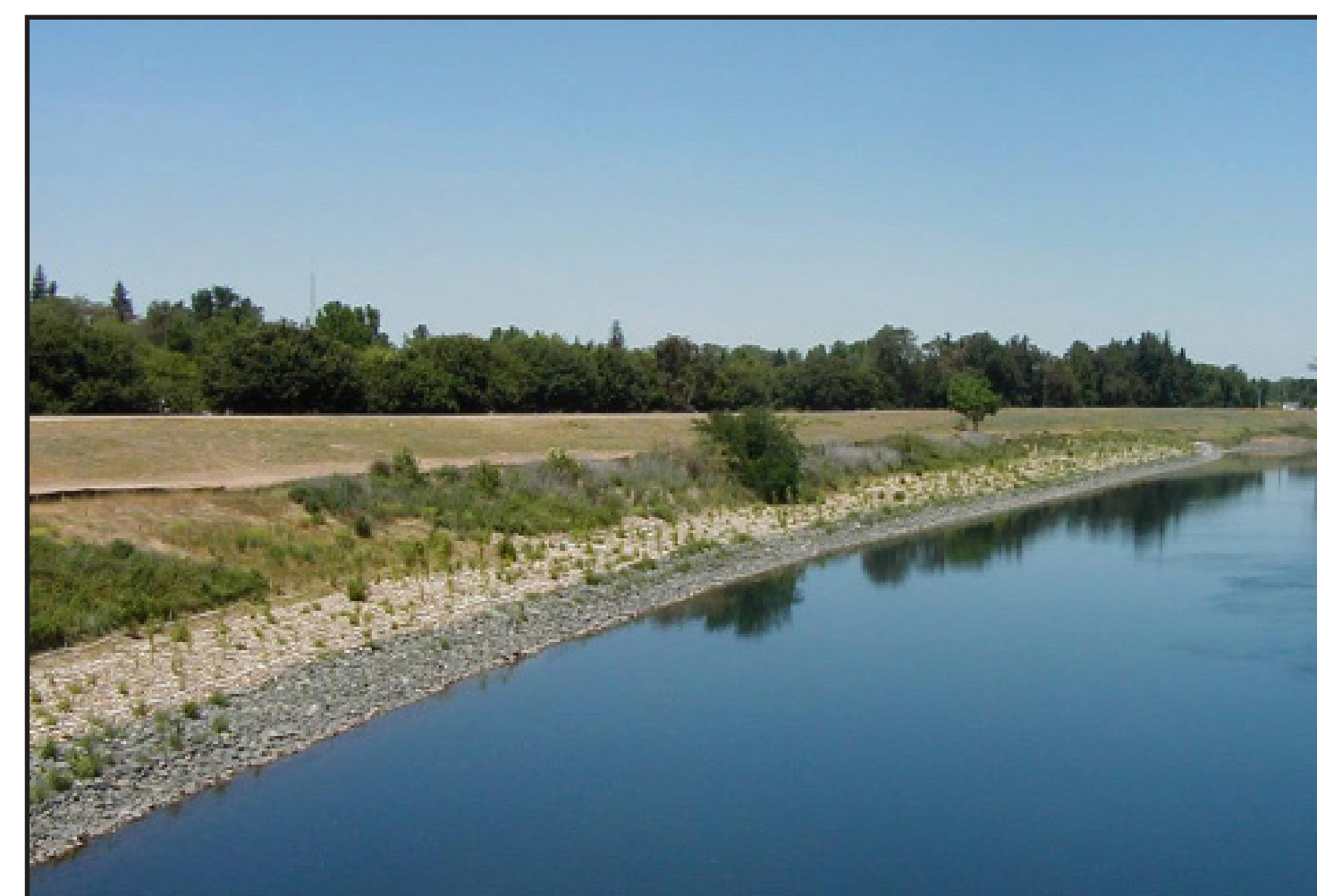
Typical bank protection as constructed at Lower American River Site 4 between Guy West bridge and H Street Bridge in 2001
