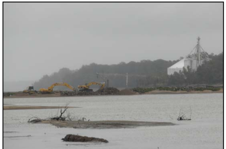
Looking upstream in the Island 70 secondary channel prior to degrading dike 1 to allow flow to inundate the channel.
