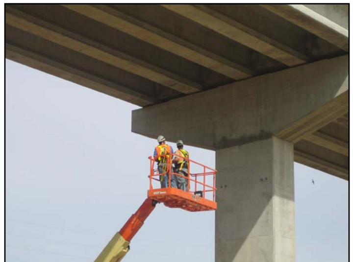
Greenwood Area Office Project Engineer, Adam Staples inspecting bridge at pre-final inspection.
