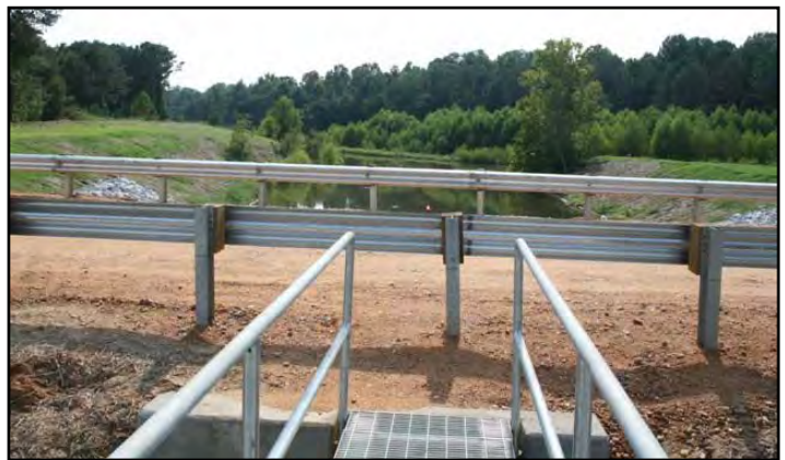
Standing on the Lower Lake Walkway Bridge looking downstream toward the emergency spillway channel
