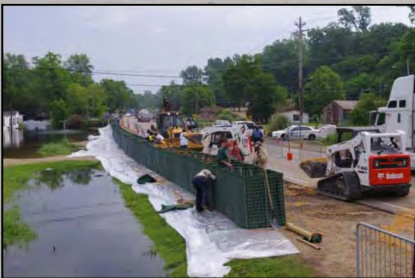
City of Vicksburg and Ergon installed Hesco Bastions on north Washington Street.
