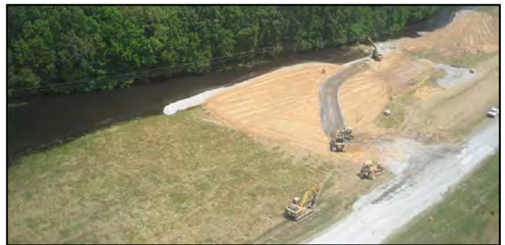
Albermarle levee slide
