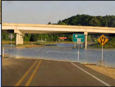
Flood water at portion of Highway 61 North
