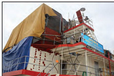
Blue tarp covers the pilot’s house portion of the Dredge.
