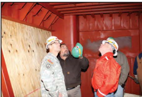
Looking up at location of leaks in the Dredge are left to right, Col Eckstein, Perry Huskey, and Patrick Chambers.
