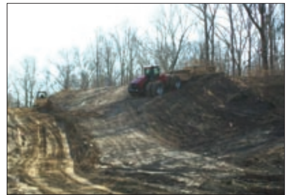
Clearing and grubbing progress on the ERDC main campus side of Wisconsin Avenue.
