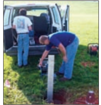
Andrew Tomlinson and Co-Op student Lance Gullet controlling the actions of the tractor and camera with monitor above the pipe during toe drain inspection at Shelbyville Dam for the St. Louis District.
