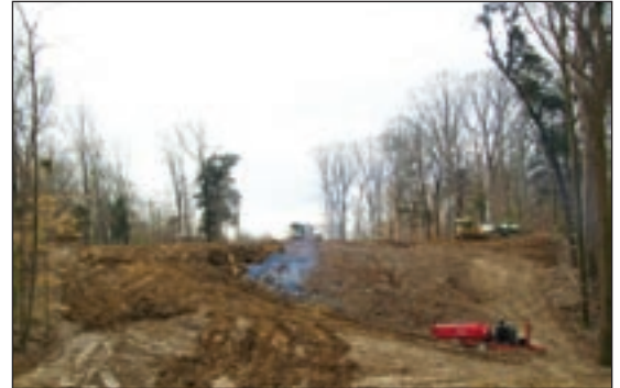
Beginning stage of the excavation and fill operations near the Information Technology Laboratory at ERDC.
