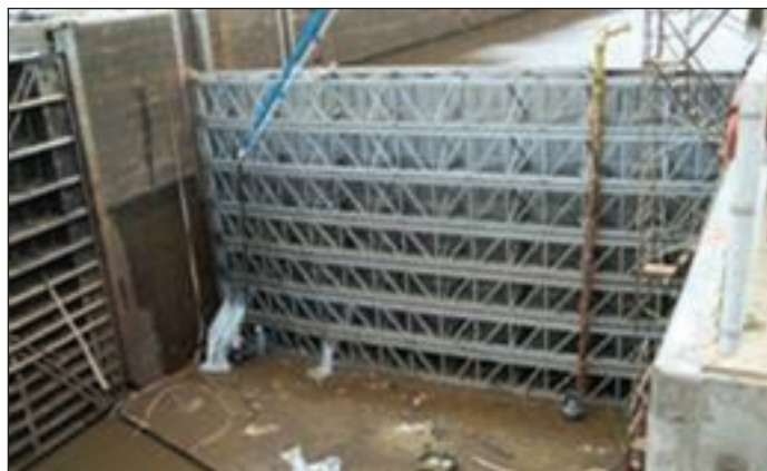
Stoplogs in place (These photos are from completed structures at the Jonesville and Columbia Lock and Dam)
