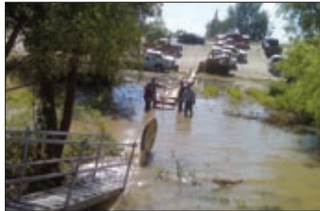
The maintenance crew uses parts from used cable reels to build a makeshift bridge to the quarter-boats.
