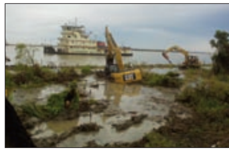
Two bulldozers free track hoe that got stuck on the river bank.
