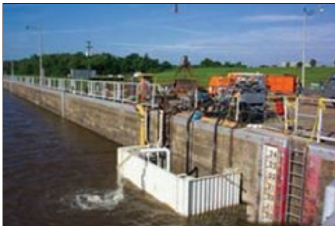
Cofferdam put in place to remove water from the lock chamber so the work can begin.
