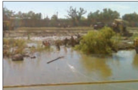
The bank crew struggles to pull cables on the flooded river bank.
