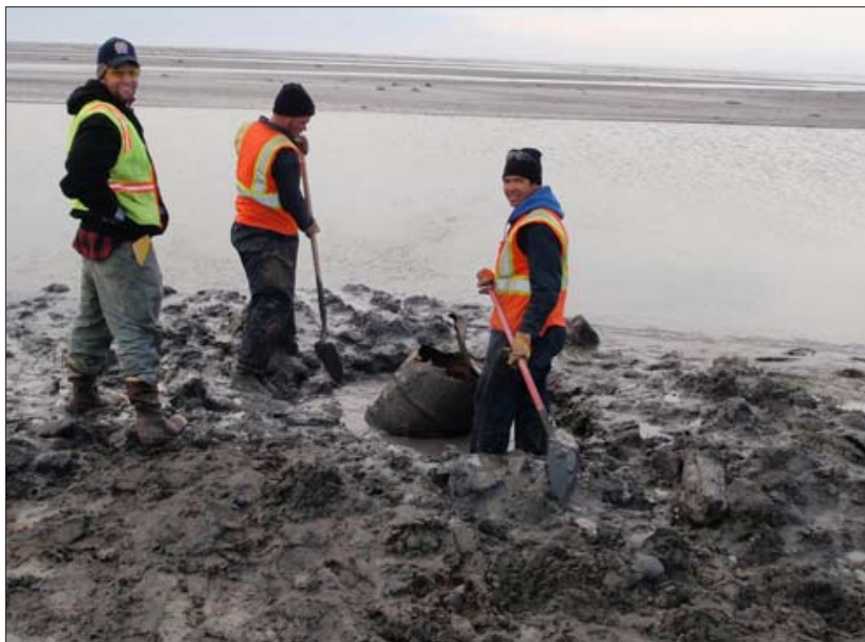
(Bottom photo) Sam Widmer (left) of Weston Solutions works with Eric Jenks (center) and Mike Flisk (right) of Marsh Creek, LLC, to retrieve a buried drum from a sand bar. All of this extraction work was done by hand. (Courtesy photos)
