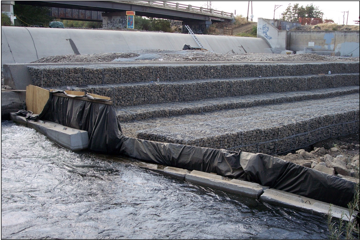
Photo 2-2: Example of a Dewatering Barrier as Installed in 2014 at Nursery Bridge. The same approximate size and location of a barrier for the 2016 work would be used.
