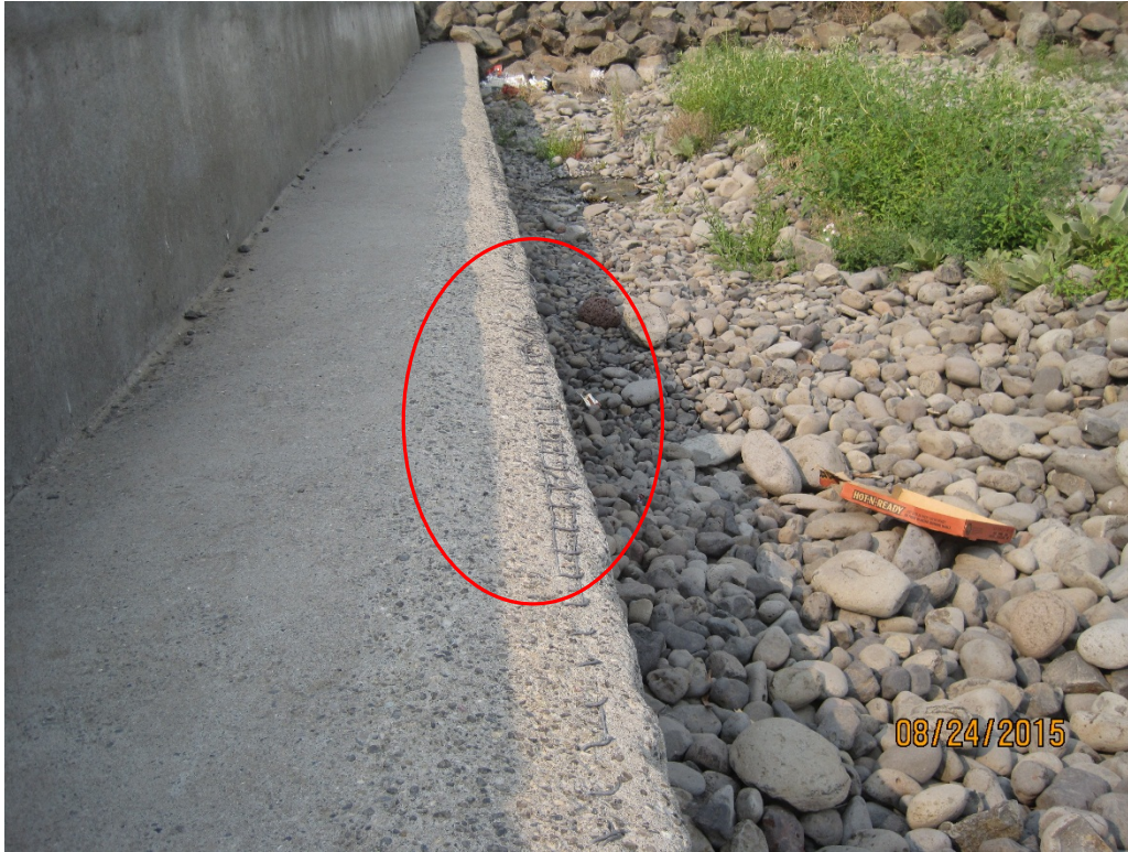
Photo 1-1: Picture Showing Damage to the Concrete (Exposed Rebar) at the Toe of the Gabion Mattress.
