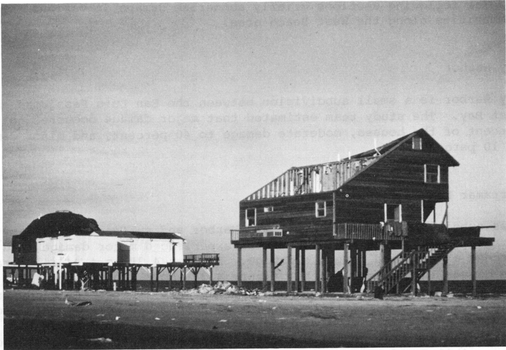
FIGURE 4.39 Example of a roof failure of a house in Terramar Beach.
