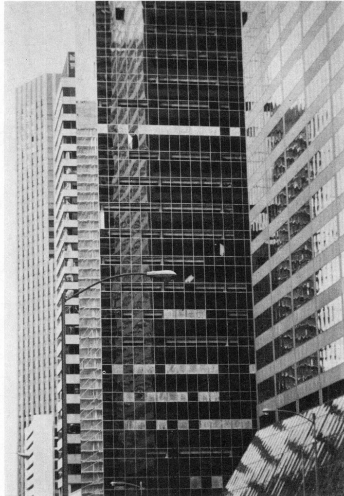
FIGURE 4.9 Glass damage to the northeast face of the Entex Building.
