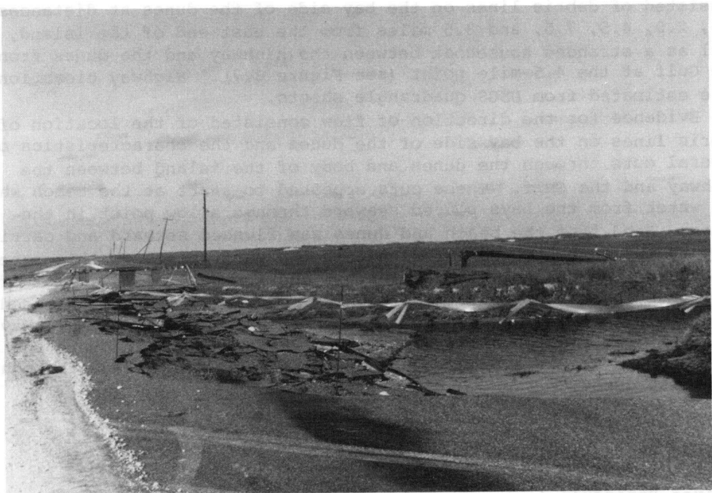
FIGURE 3.8 Washout channel looking south toward the Gulf about 7 miles west of San Luis Pass on Follets Island.
