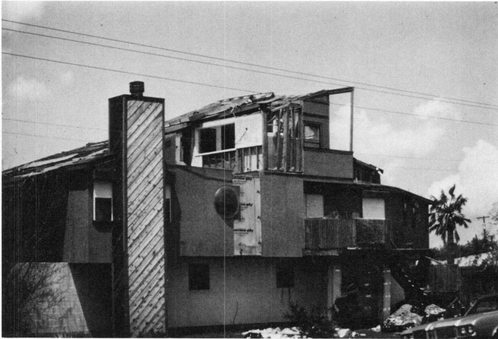
FIGURE 4.63 Roof damage to a condominium in Texas City.
