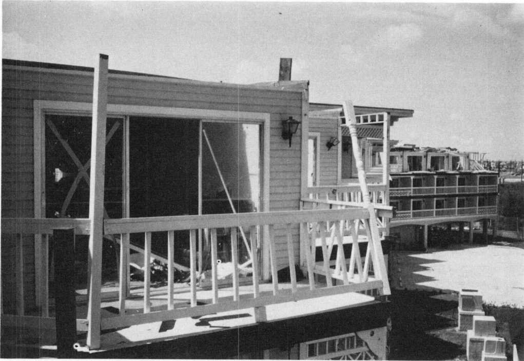
FIGURE 4.30 Closeup of a damaged unit in the Victoria Hotel.
