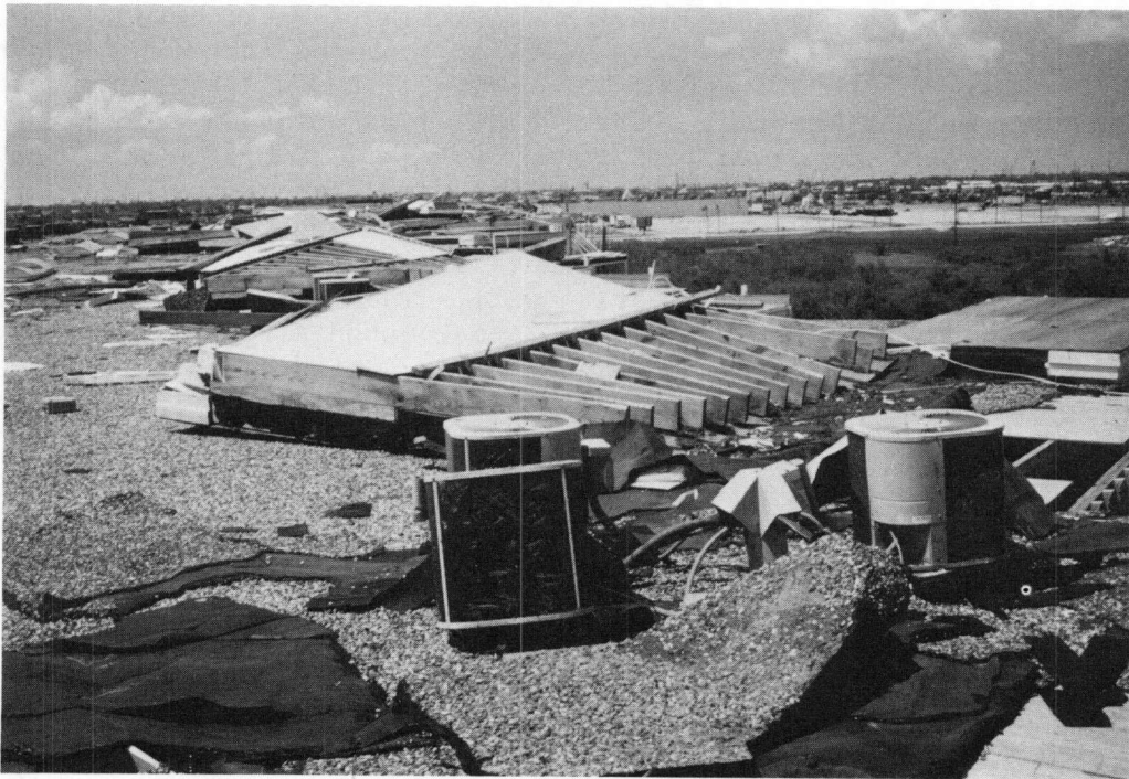
FIGURE 4.31 General view of the roof of the Victoria Hotel, showing damaged overhangs that landed on the roof.
