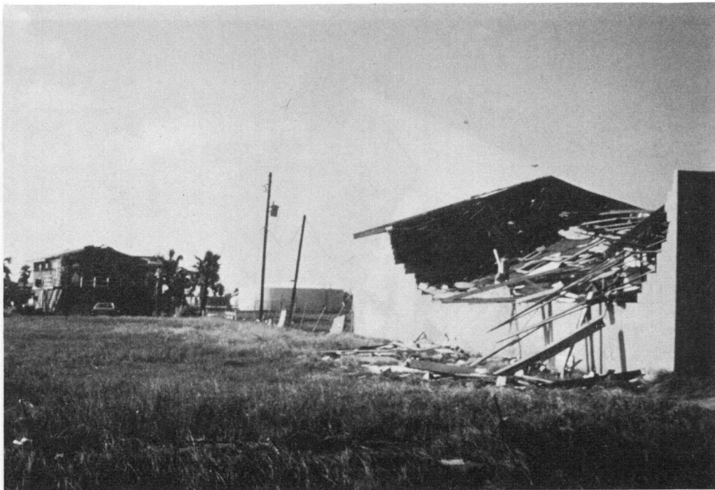
FIGURE 4.50 Damage to a large commercial warehouse building.
