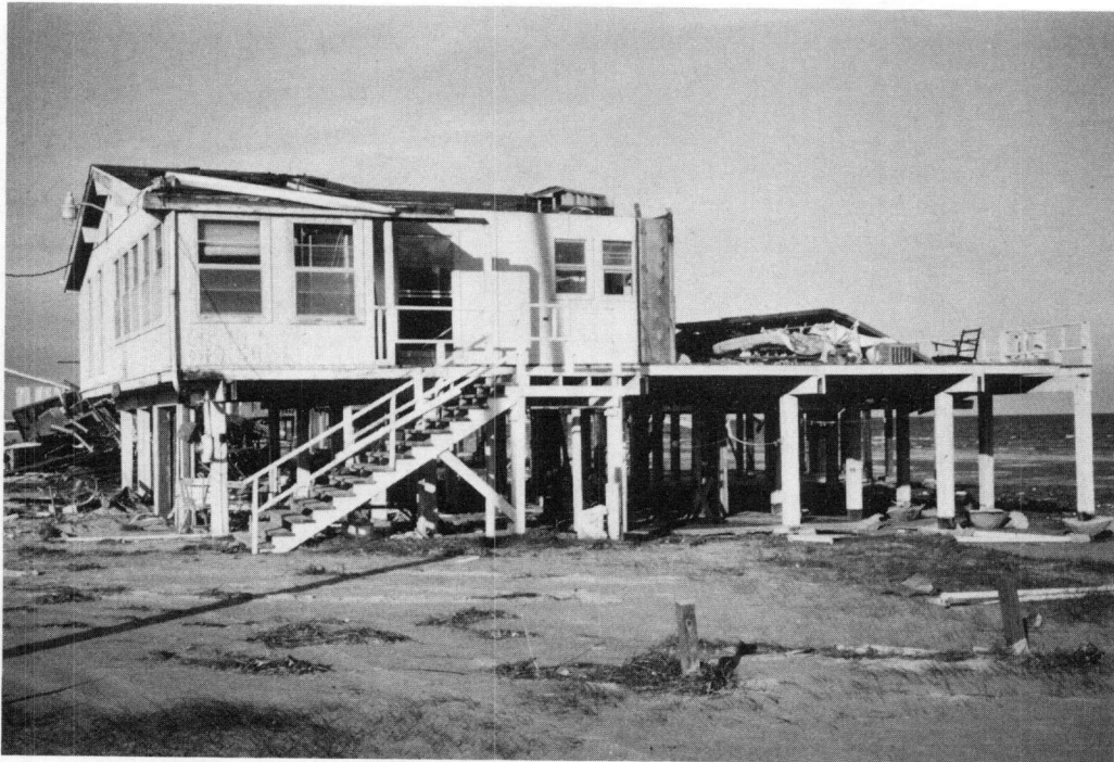
FIGURE 4.42 Typical example of partial collapse of a large house in Terramar Beach.
