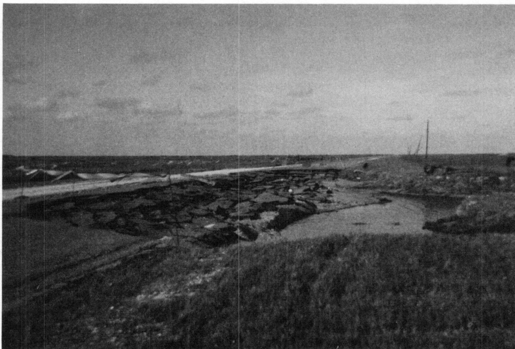
FIGURE 5.2 Typical undercut of roadbed on San Luis Pass Road, Follets Island.
