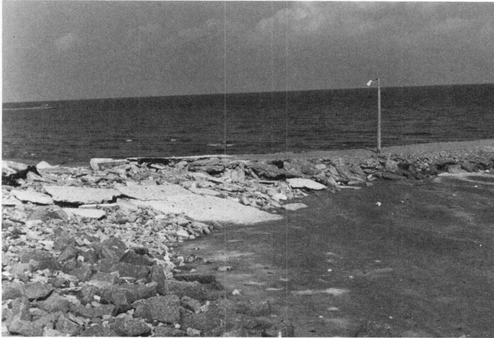
FIGURE 4.55 Damage to groin in front of the Galveston seawall.
