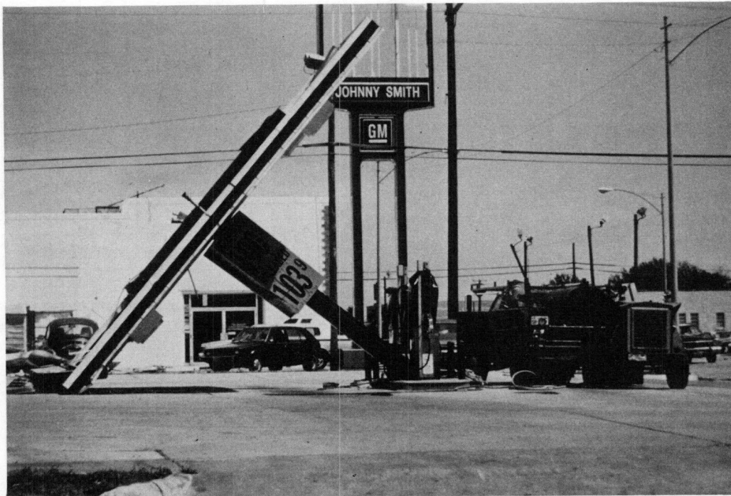
FIGURE 4.15 Example of failure of a roof support pedestal column.
