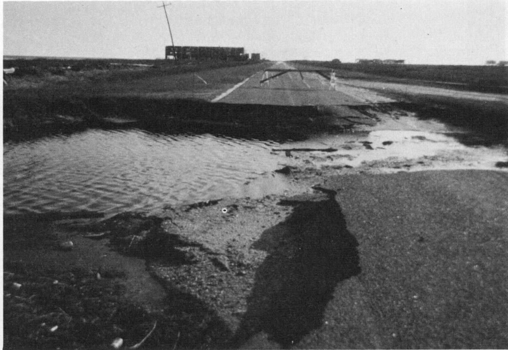
FIGURE 5.3 Total washout of shoulder and road on San Luis Pass Road, Follets Island.
