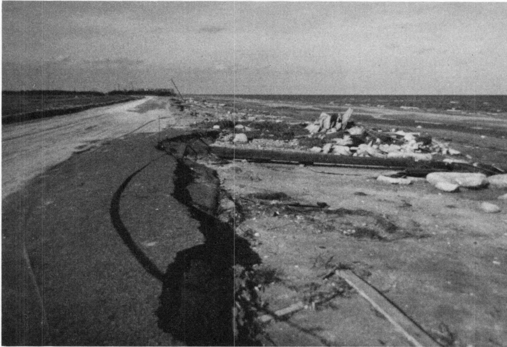
FIGURE 5.1 Typical washout of shoulder on San Luis Pass Road, Follets Island.
