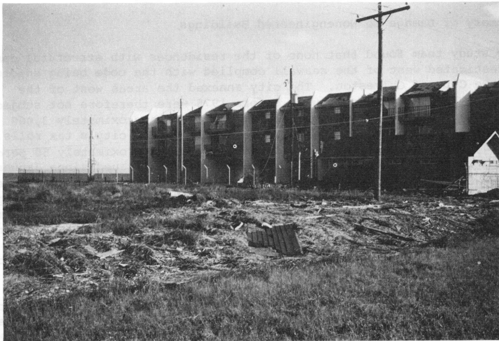
FIGURE 4.52 Damage to the roof and erosion around foundations of condominium units on the west side of San Luis Pass.
