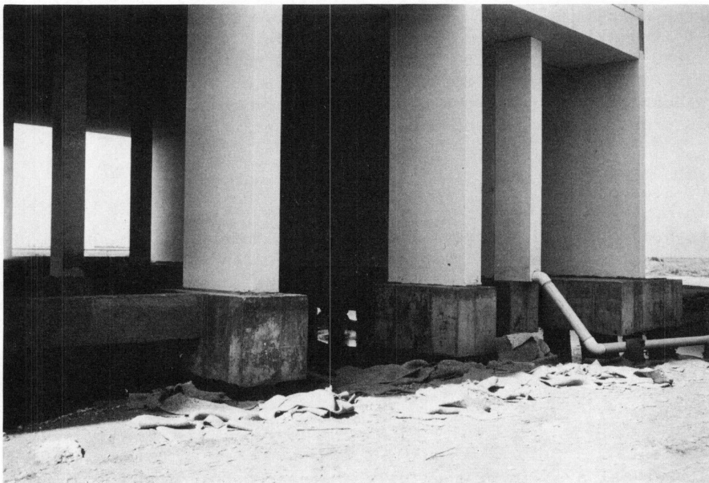
FIGURE 4.20 Erosion around the foundation of the Galvestonian.
