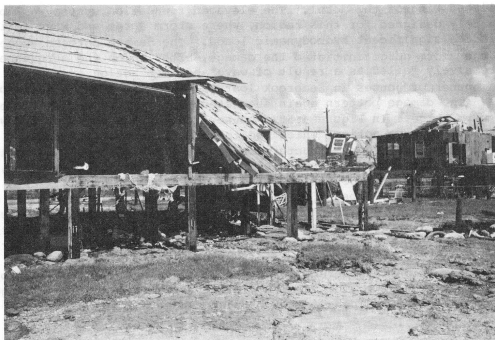
FIGURE 4.58 Bayfront house with a collapsed roof.
