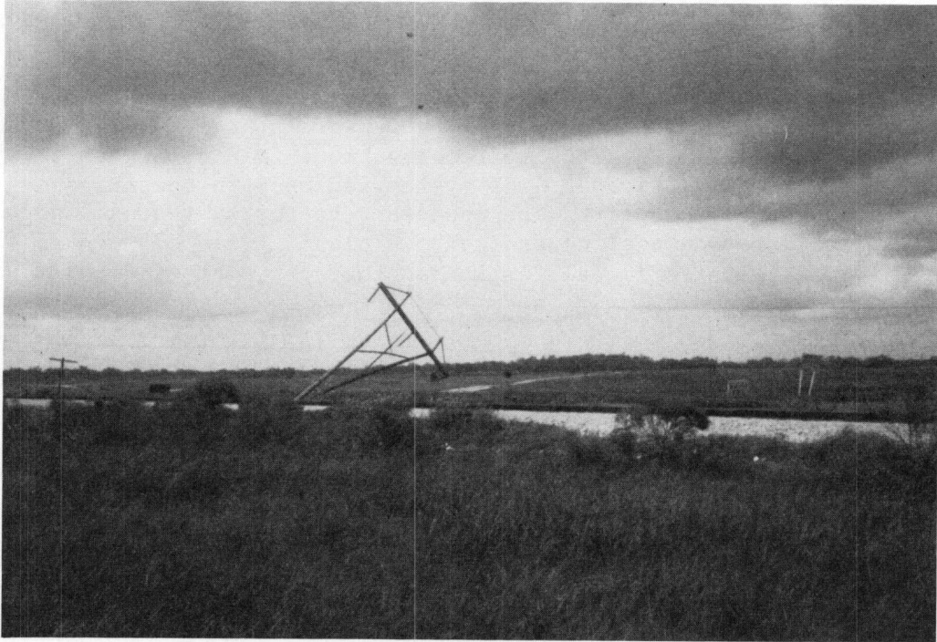
FIGURE 5.6 Failure of primary power pole near Highway 146 south of Bay City.
