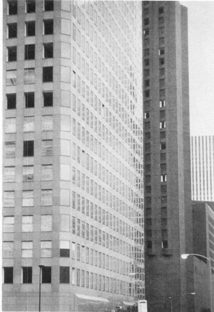
FIGURE 4.7 Window damage to the Hyatt Regency Hotel (the building in the background).
