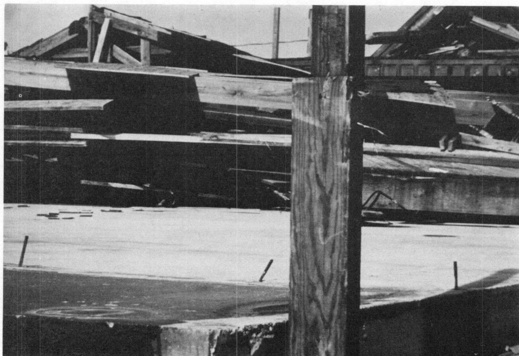
FIGURE 4.60 House washed away from its foundation slab by storm surge.
