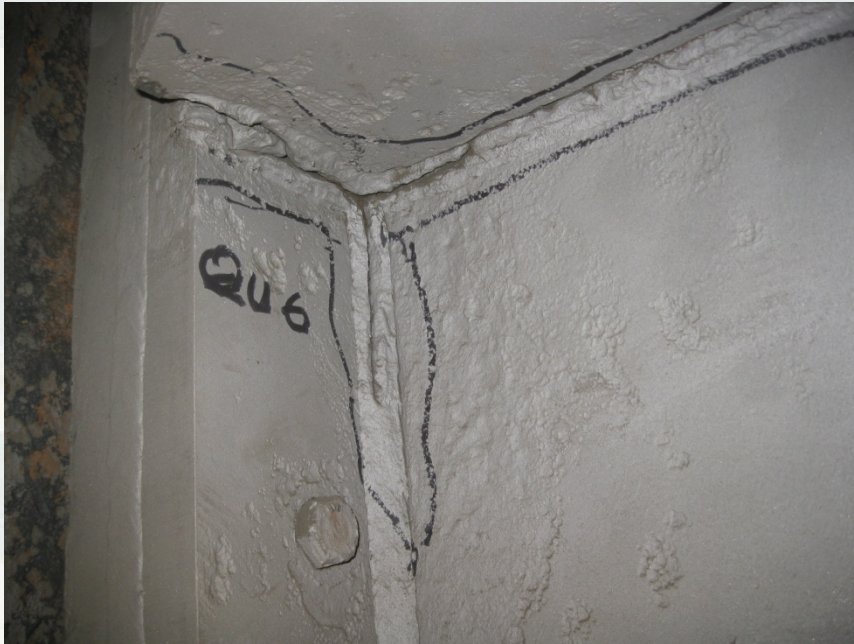
Cracks at Upstream Quoin Block
