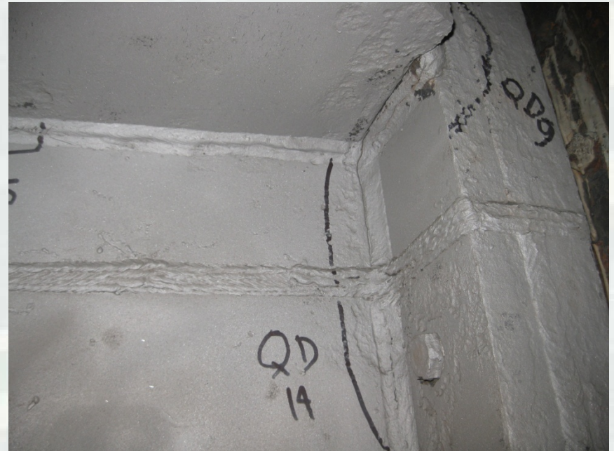
Cracks at Downstream Quoin Block
