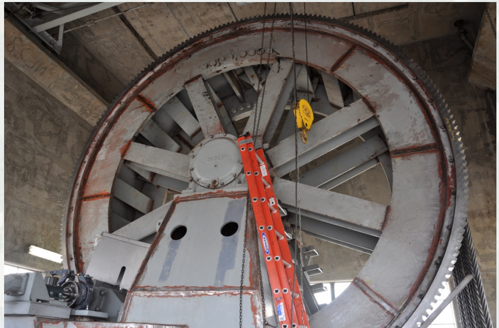
Hoist Friction Sheave – 18 ft diameter
