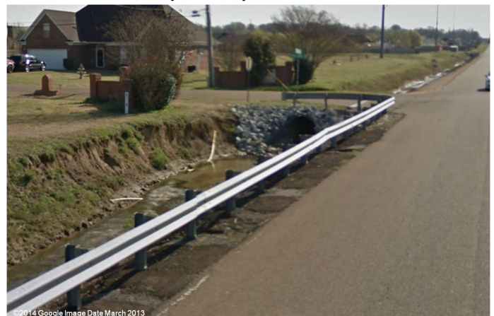
Erosion along Stateline Road, Southaven, MS
