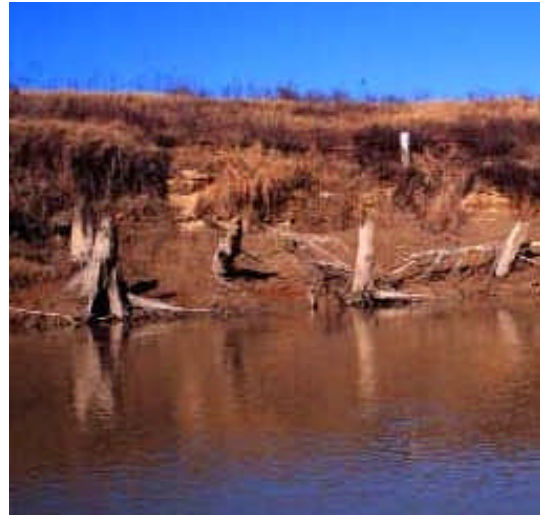
Figure 7. Tree stumps and a deadman anchor, exposed by erosion on a recently channelized river
