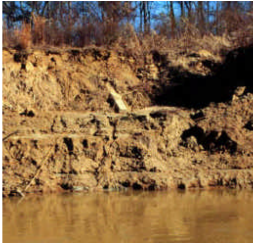
Figure 4. Deadman anchor that failed due to bank erosion
