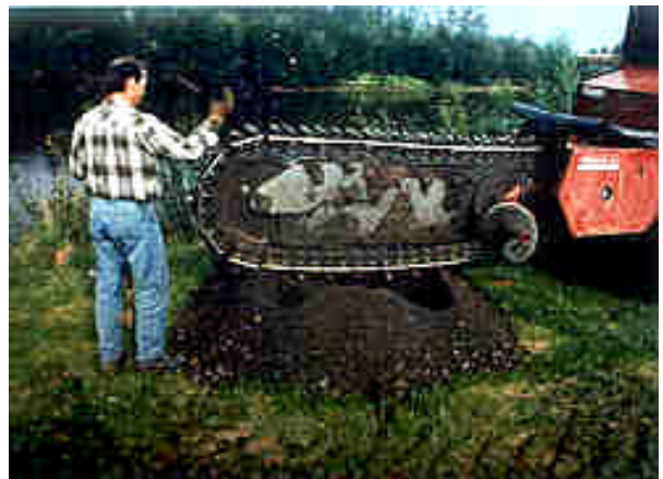
Figure 6. Ditches used to run cables from LWD to anchors on the top bank
