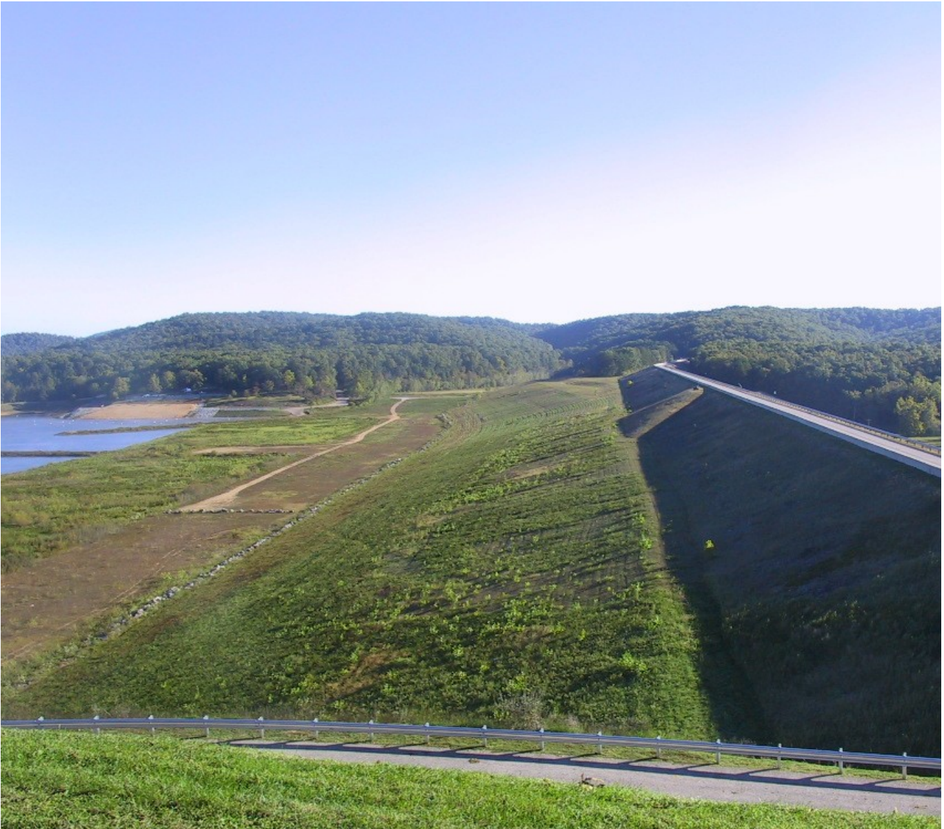
FIGURE 8-2 Existing Structure with Upstream Impervious Blanket on Face of Dam, & Seepage Berm to the Left
