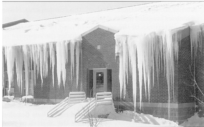
Figure 1. Severe icings along the eaves of a poorly ventilated roof.
