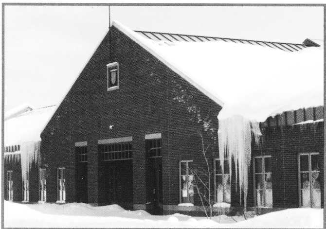
Figure 3: Minor icings occurred along the eaves of this roof and problematic icings developed at the base of valleys.
