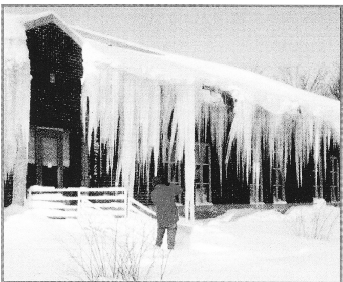
Figure 4: Severe, problematic icings developed all along the eaves of this dining facility.
