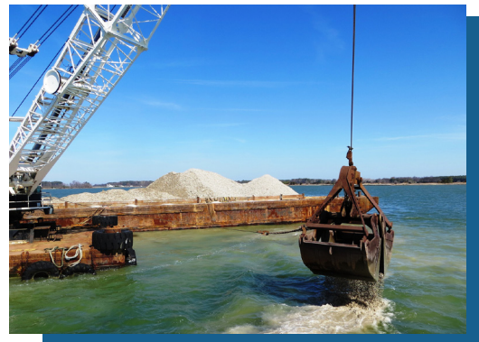
The U.S. Army Corps of Engineers, Baltimore District, places shell to restore oyster reefs in the Chesapeake Bay tributary of Harris Creek, April 1, 2015. The shell comes from processing plants in the mid-Atlantic region and is permitted to be imported and placed in the river. (U.S. Army Photo by Sean Fritzges)
