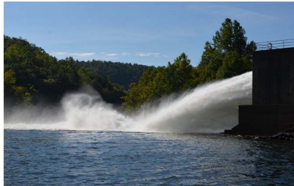
Summersville Dam Fixed Cone Valves
