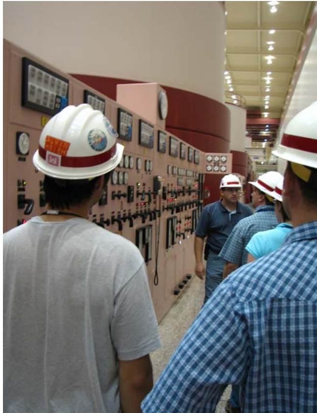
EITs OBSERVE A GOVERNOR CONTROL PANEL AT CHIEF JOSEPH DAM, WASHINGTON
