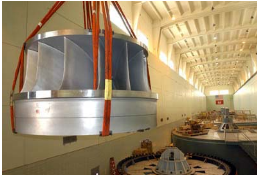
A NEW FRANCIS TURBINE RUNNER INSTALLATION AT J. STROM THURMOND DAM, SOUTH CAROLINA
