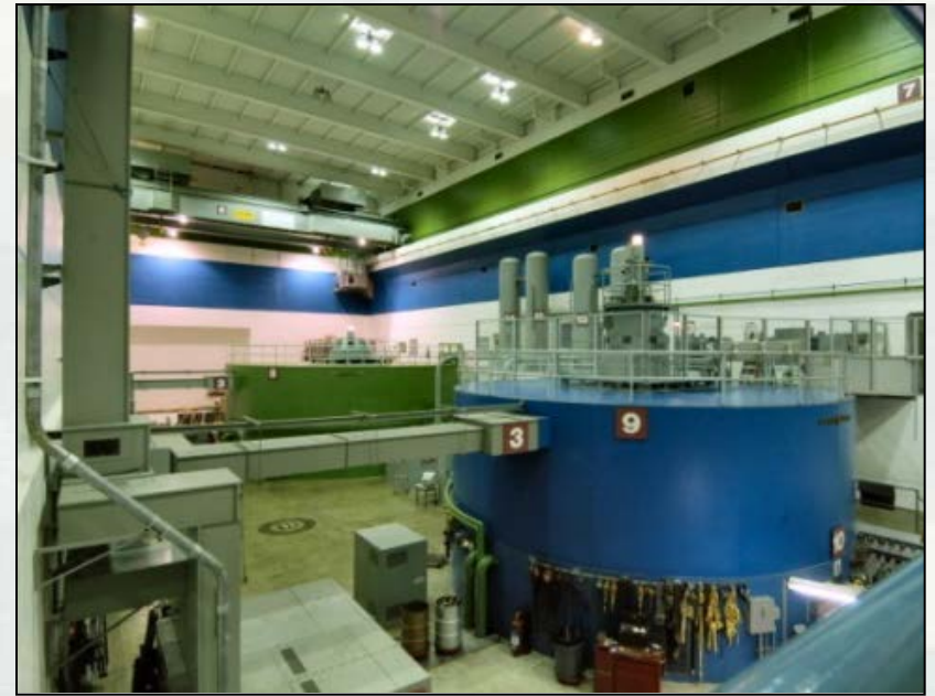
Hydropower plant, Clarence Cannon Dam, Monroe City, Missouri.
