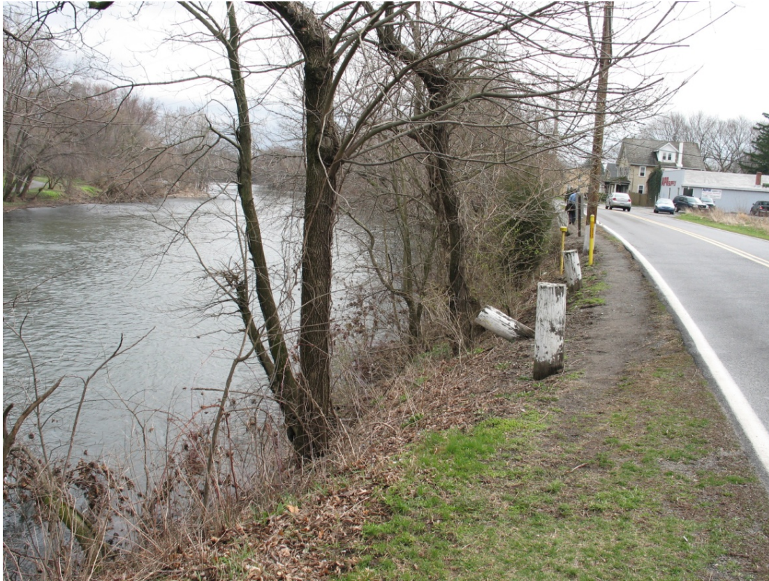
Figure 5. Another view of project area with failing streambank and infrastructure (Photo 2008).
