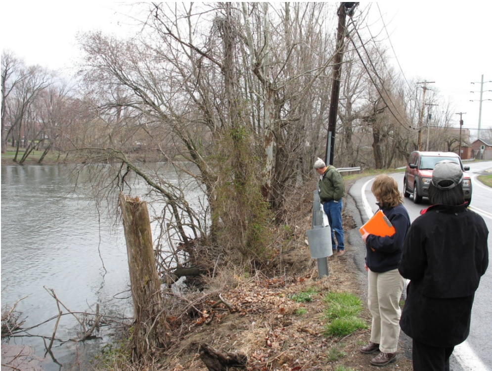
Figure 4. View of project area with the failing streambank (Photo 2008).
