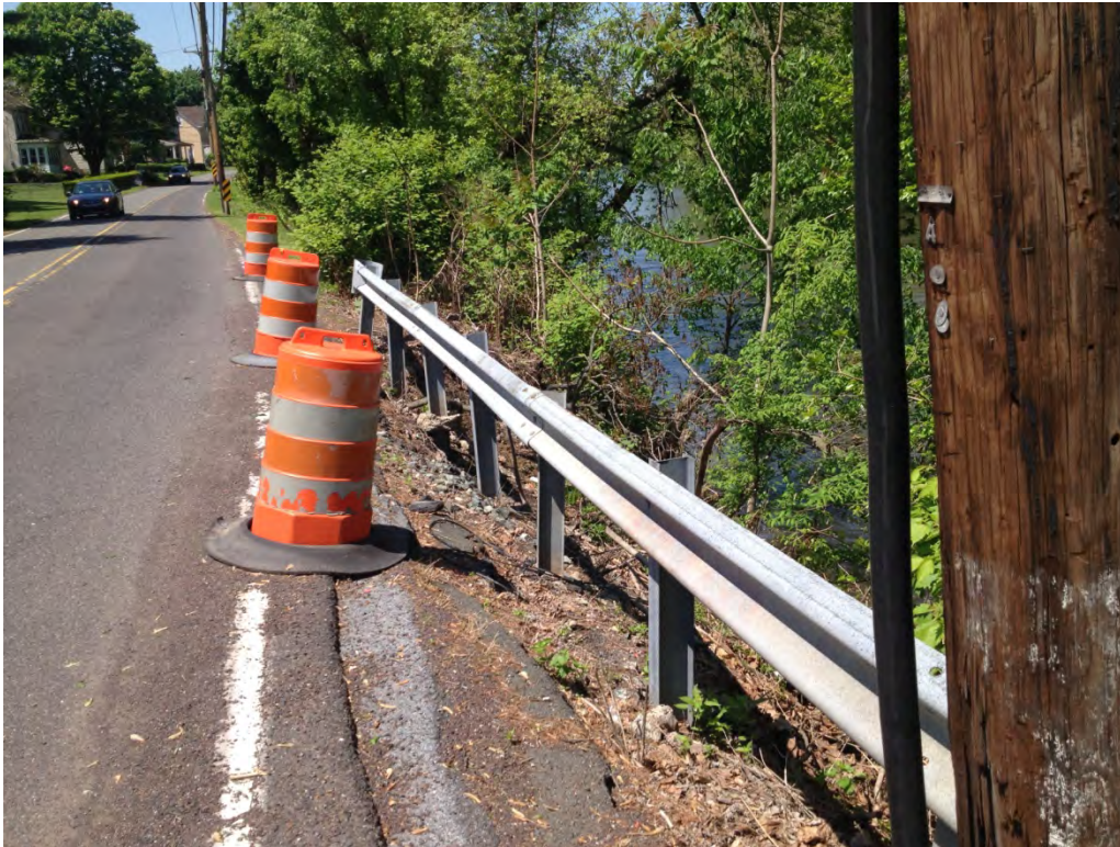
Figure 4. View of project area with the failing streambank (Photo – May 2014).
