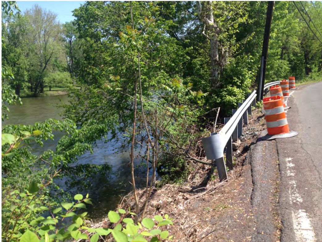
Figure 5. Another view of project area with failing streambank and infrastructure (Photo – May 2014).
