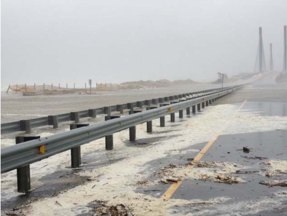
Photo 1: State Route 1 and Indian River Bridge during a recent storm (March 6, 2013).
