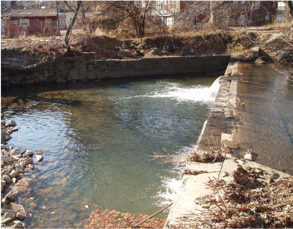
Figure 3. Woodland Dam shown from the bank adjacent to the Blue Bell Inn.
