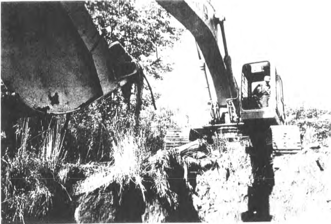
PHOTOGRAPH 54 - 9/17/97 Thick lubricant oozing from drum in trackhoe bucket
