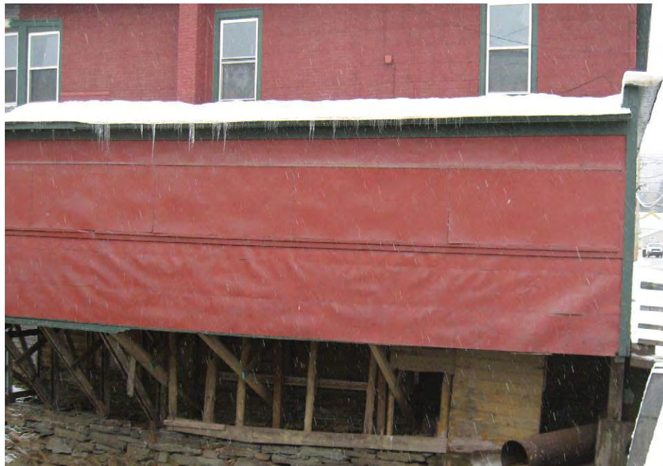
Photograph 20: Building (A030) and stone foundation in south quadrant of Area 7. Little Beaver Kill is channelized along the stone foundation. An out-spill pipe is located just below the building at the juncture of the foundation and the bridge abutment. Facing southwest (February 2010).
