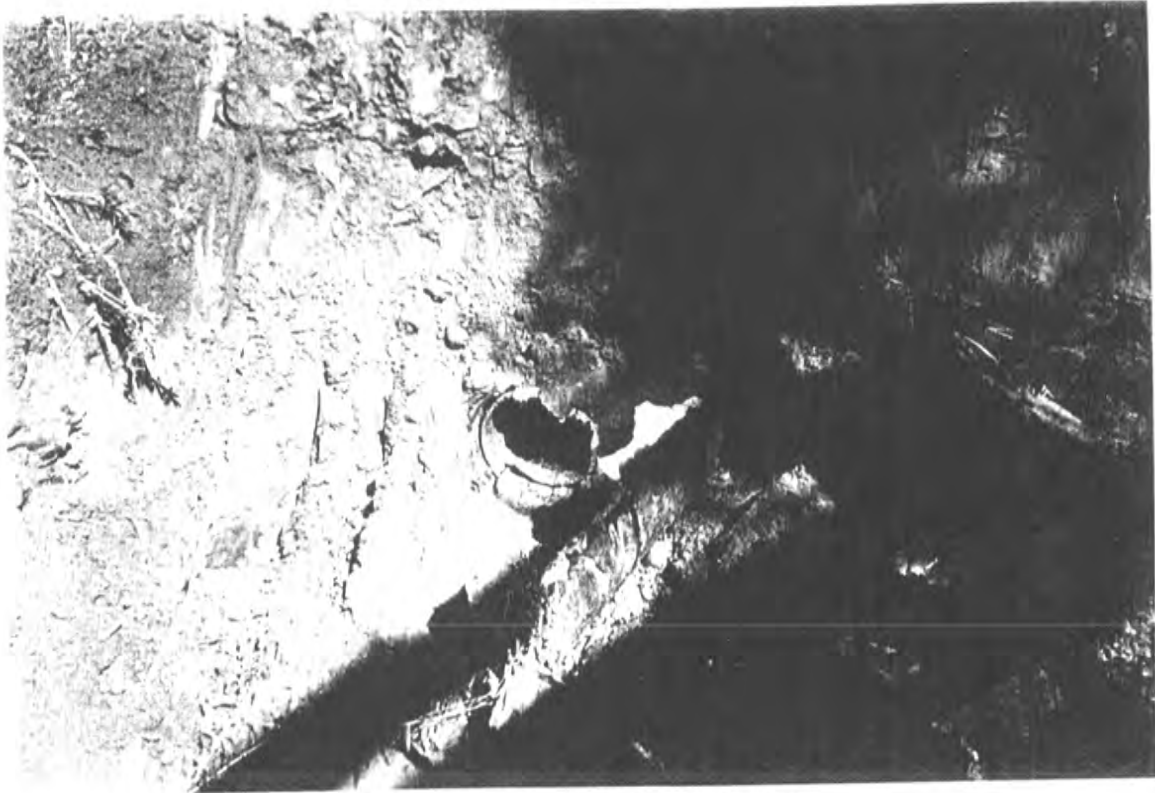
PHOTOGRAPH 3 - 9/15/97 Broken sewer pipe (between O-75 & P-75)
