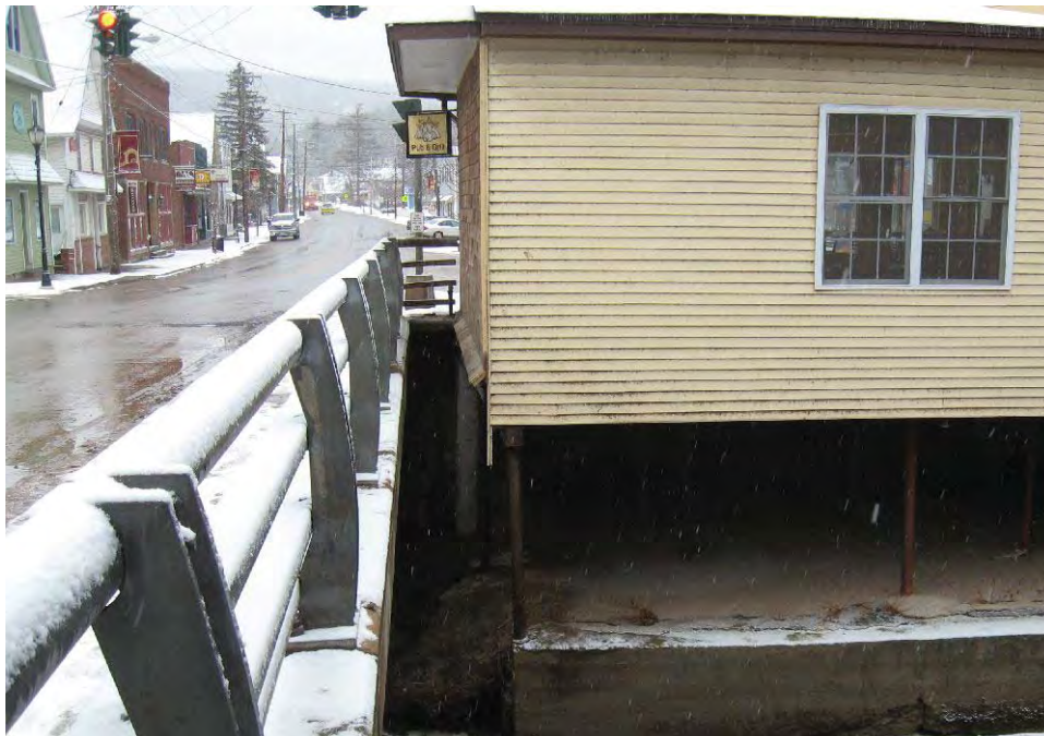
Photograph 22: Building (A029) and stone foundation in east quadrant of Area 7. Little Beaver Kill is channelized along the stone and cement foundation. Facing northeast (February 2010).
