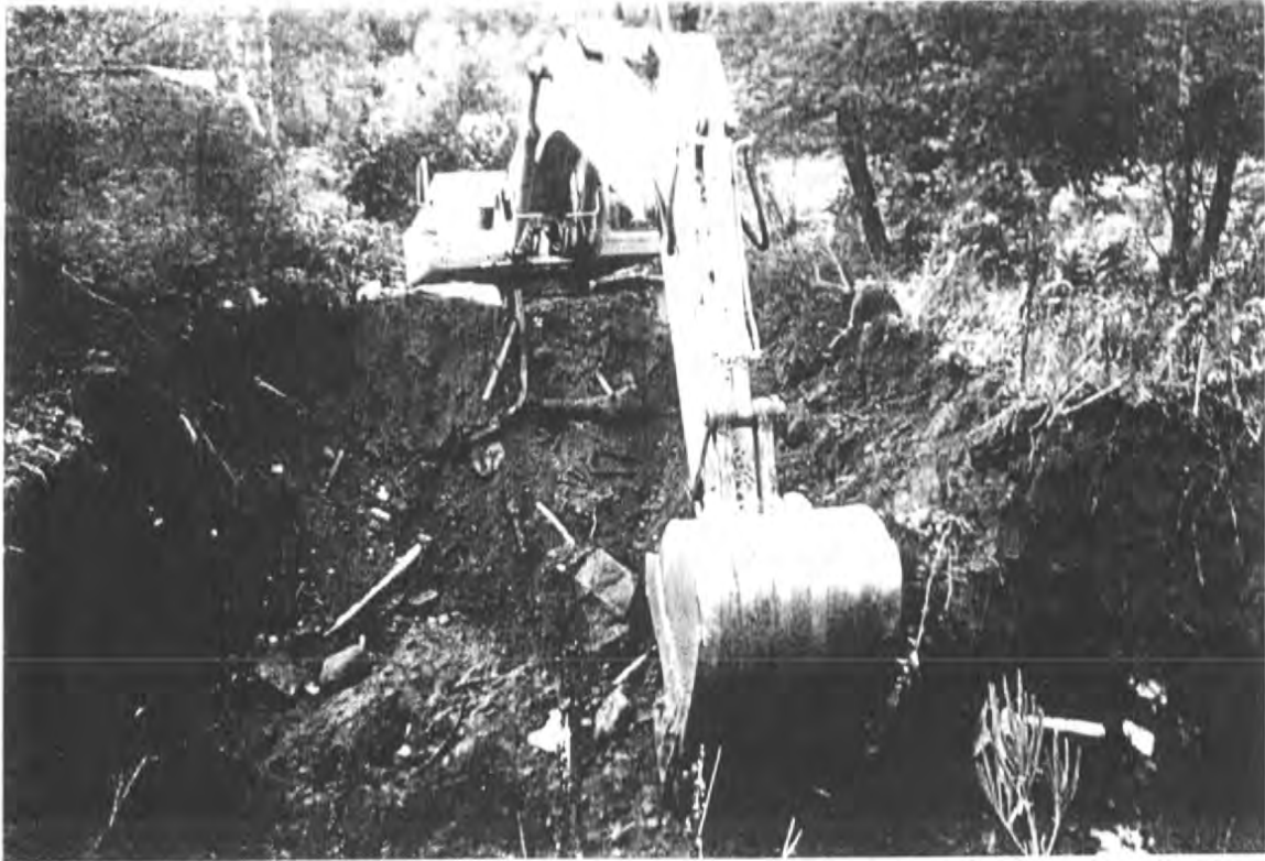
PHOTOGRAPH 9 - 9/15/97 Metal debri, pipes (East of D-400)
