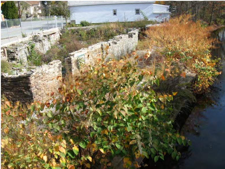
Figure 11.2 - Remnant of Building on ROB Upstream of Main Street Bridge after Fire
