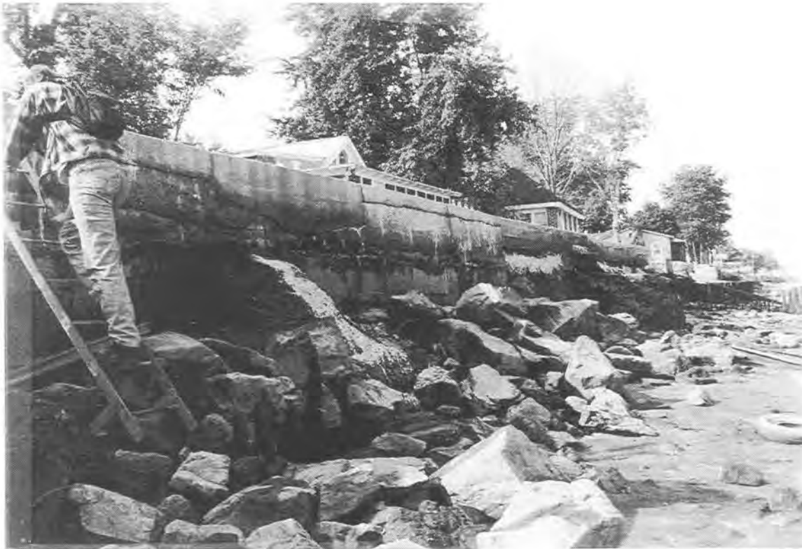
Photo #13: Remains of a failed wall fronting a deteriorated concrete vertical wall.
