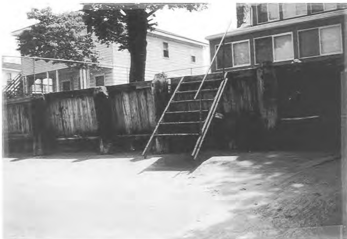
Photo #18: Northern 1/3 of beach. Note the vertical loss of beach from the bottom of the ladder which occurred relatively recently.
