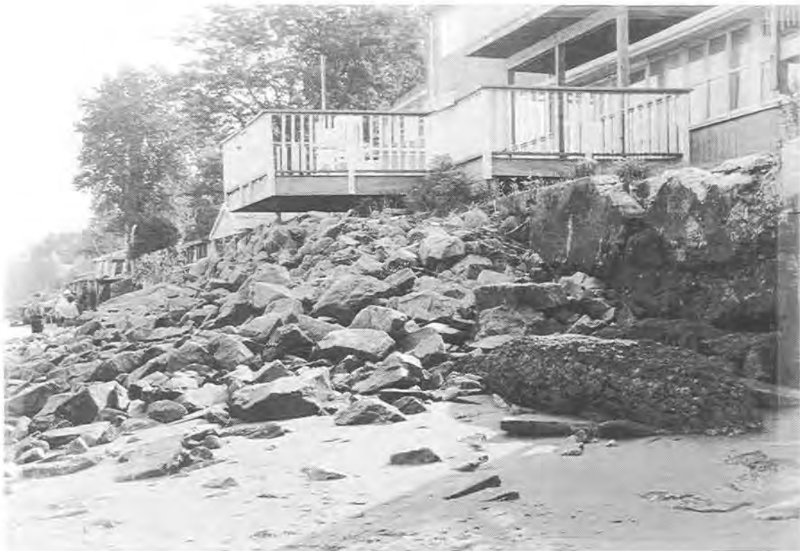
Photo #11: Southern 1/3 of beach. Stone revetment recently placed by a local resident in front of a deteriorated concrete wall. Note the condition of the concrete wall on the right (i.e. substantial protection next to deteriorated protection allows flanking to occur – no consistent protection).
