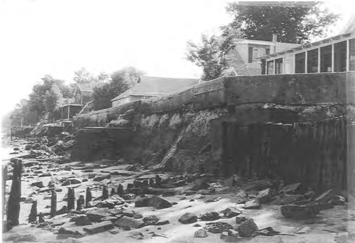
Photo #12: Southern 1/3 of beach. Deteriorated concrete wall and timber bulkhead. Remains of a timber groin in the foreground.
