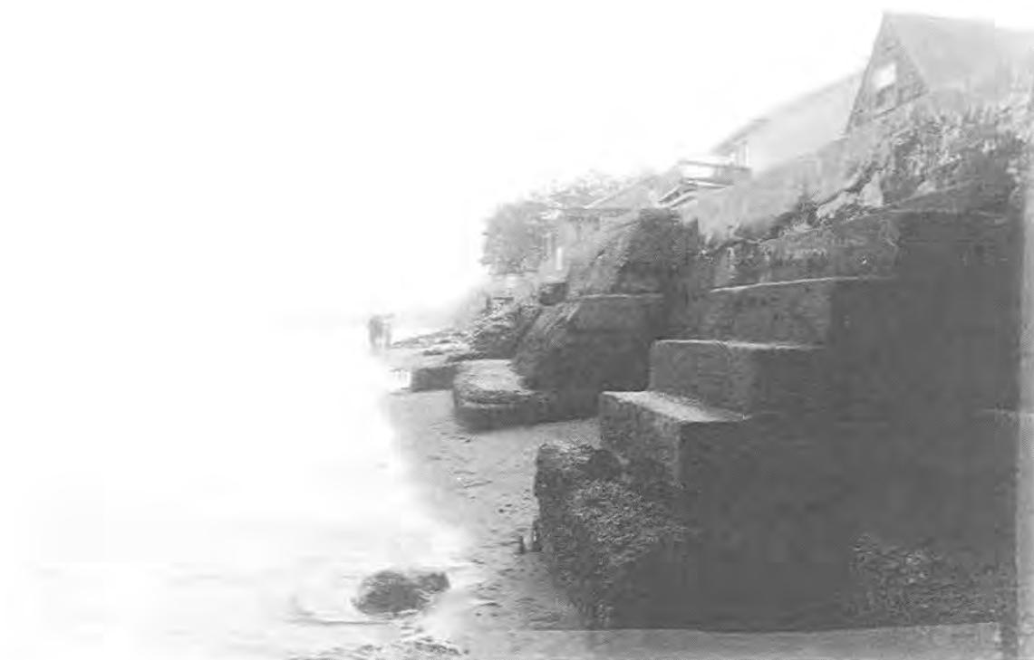
Photo #10: Southern 1/3 of beach. Note concrete steps adjacent to the wall. These steps were constructed during a later time period following a vertical drop in the beach elevation.
