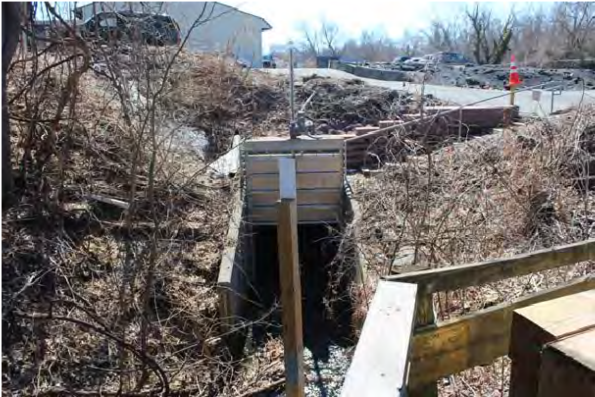
Figure 3-7: FEMA Mitigation Project (sluce gate)
