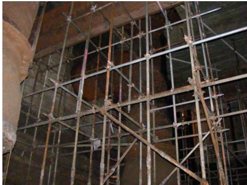
Pump Station #2 discharge pipes supported by scaffolding
