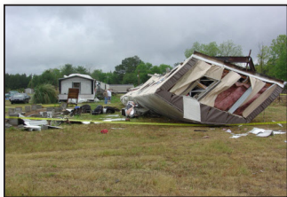
A mobile home was destroyed by a tornado. Photo credit: NOAA/National Weather Service
