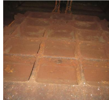
Sluice Gate in need of repairs
