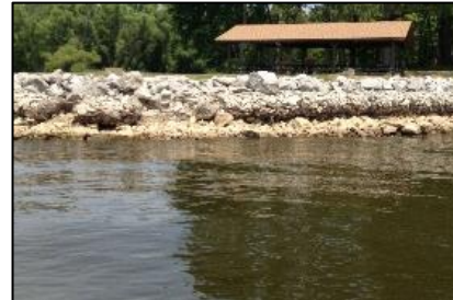
Recreation area shoreline damage due to flooding
