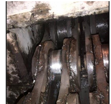
Failed Liftgate Hoisting Rollers at Locks 27
