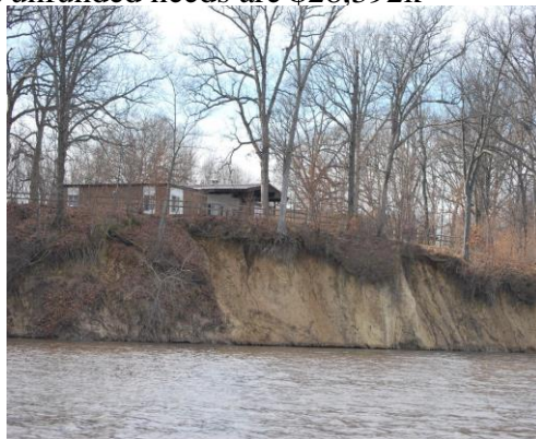
Erosion occurring on many banklines at project (January 2016)
