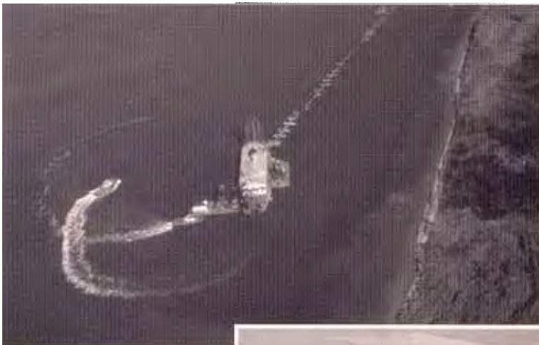
Above: Dredging activity on the GIWW keeps the waterway to its 12-foot depth.
