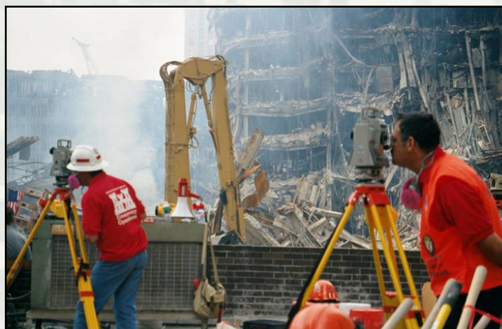
Corps of Engineers structural experts kept a constant watch on the heavily damaged structures surrounding Ground Zero, to look for any signs they might collapse while recovery efforts were taking place. (File Photo)
