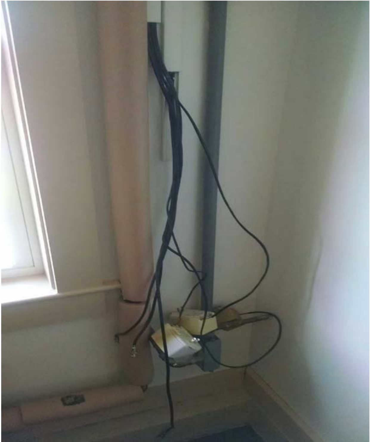
Informational Photo Number 2: Existing coaxial cable inside Office.
