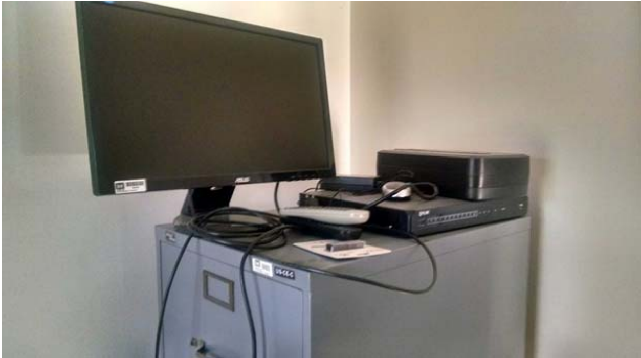
Informational Photo Number 1: Existing DVR System (Non-functioning).
