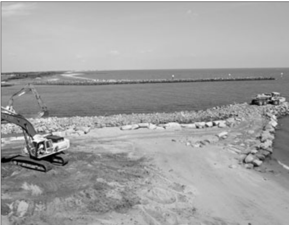
Construction of the Roosevelt Inlet/Lewes Beach Project (Del.) near the mouth of the Delaware Bay
