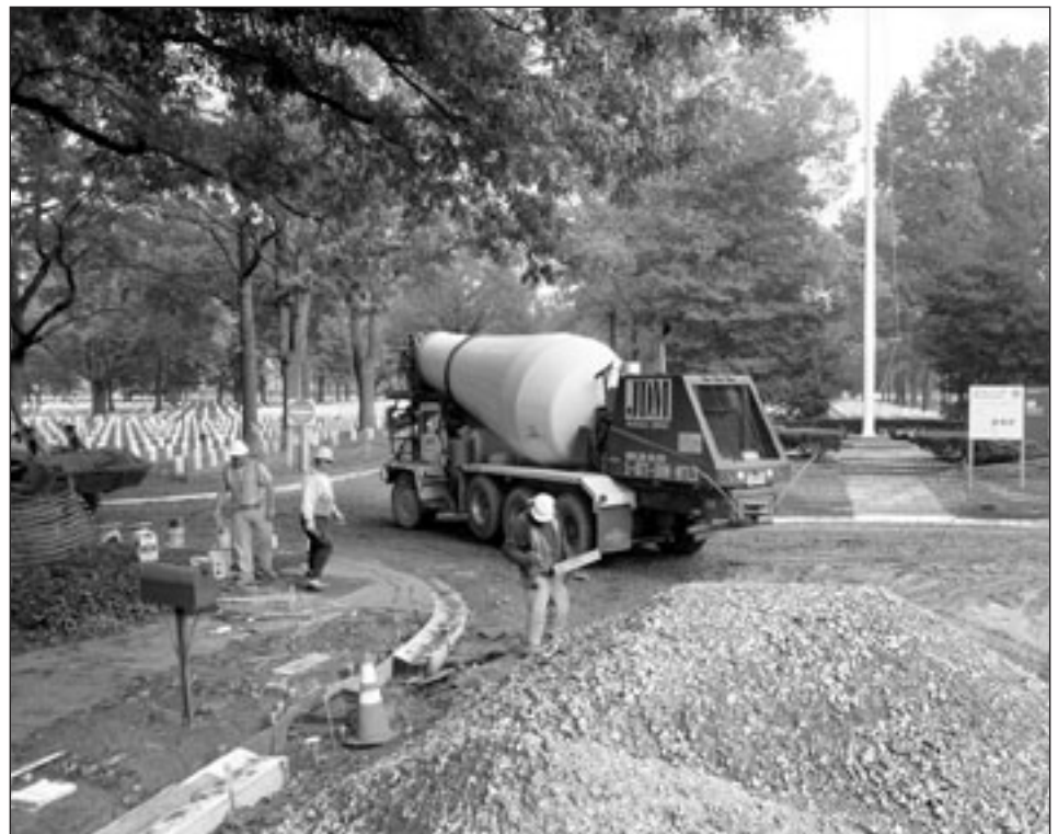
Another federal customer was the U.S. Department of Veterans Affairs, which engaged the District's services to repair and upgrade the roads inside Beverly (N.J.) National Cemetery
