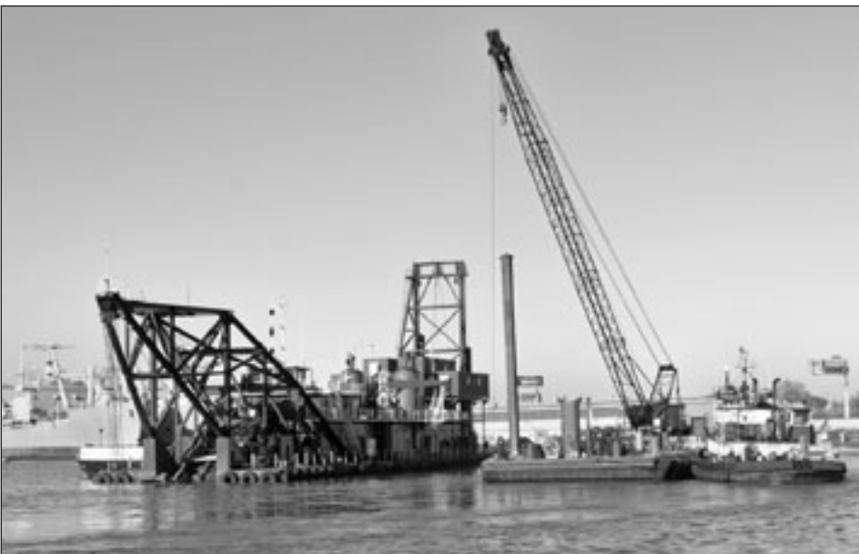
Dredging the “Reserve Basin” at the mouth of the Schuylkill River for the Department of the Navy
