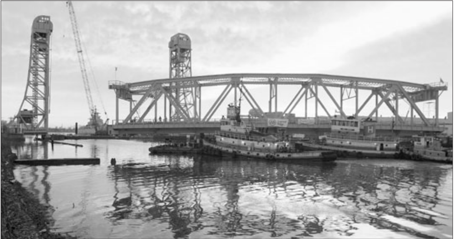
Float-in of the renovated main span for the Coast Guard's Vertical Lift Bridge project at the former Philadelphia Naval Shipyard (above)
