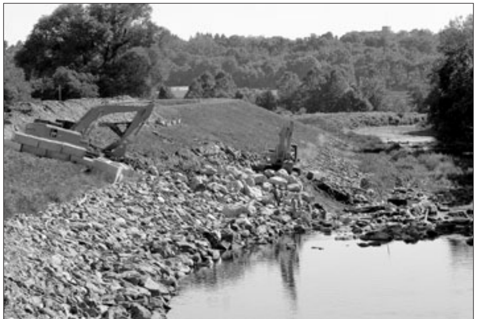
Repairs to a storm-damaged levee at Stroudsburg, Pa., under the Public Law 84-99 Rehabilitation & Inspection Program
