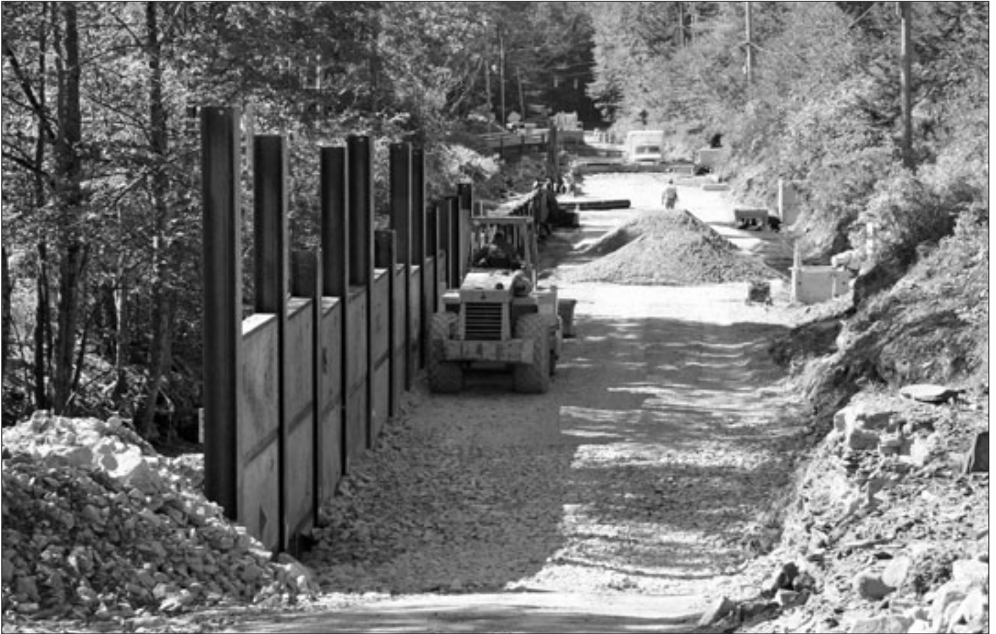
Construction of a streambank erosion control project along Basket Creek in Sullivan County, N.Y.
