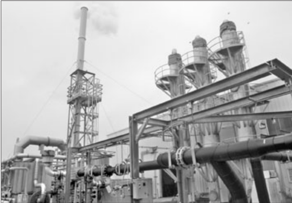
The batch flushing and treatment plant at the Lipari Landfill site
