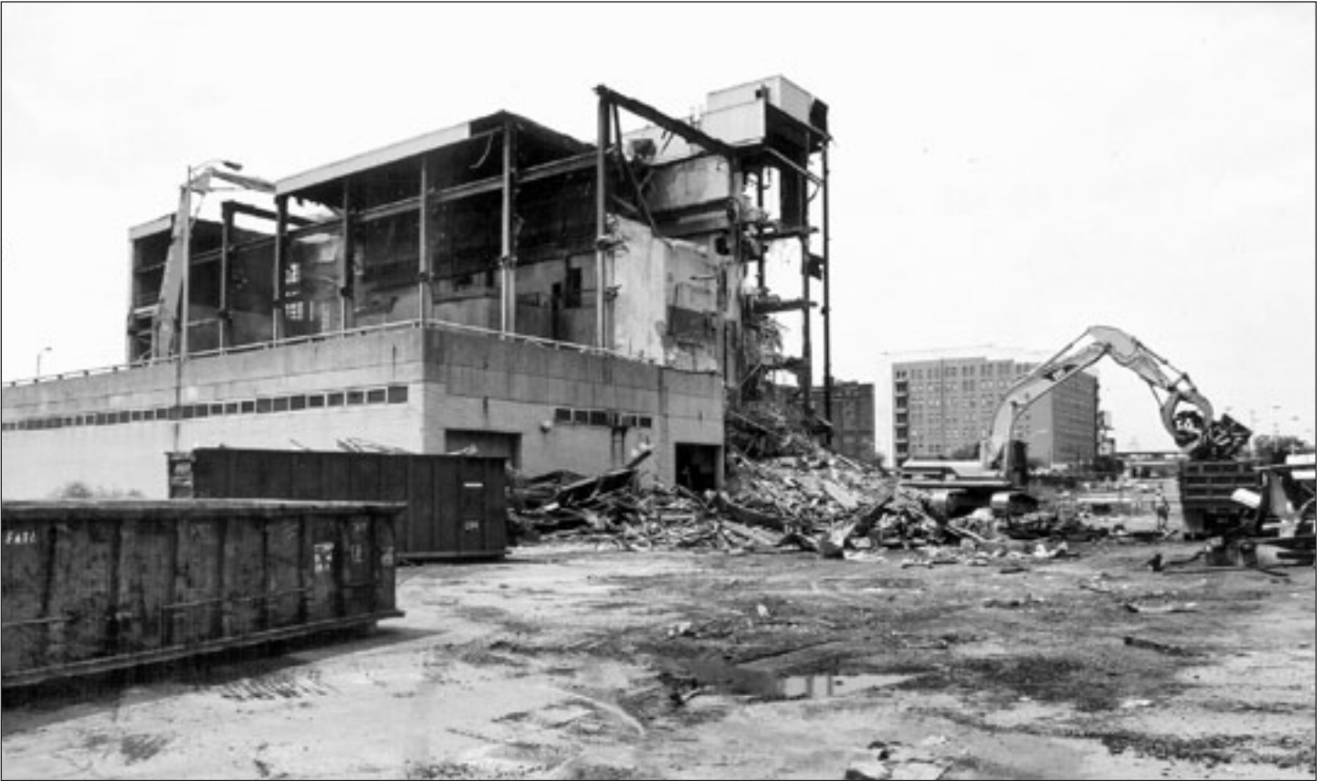
Demolition of the East Central Incinerator along Philadelphia's Penn's Landing waterfront area
