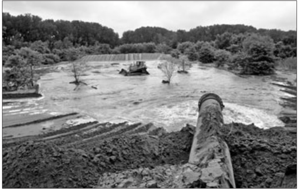
Dredge pumpout at Palmyra Cove, where part of the original disposal area was converted into a nature center
