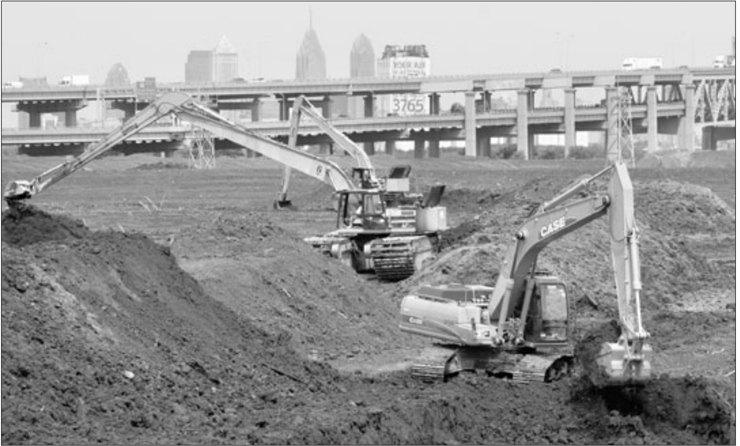
One of the district's federally owned and operated confined disposal facilities for dredged material at Fort Mifflin, Pa.
