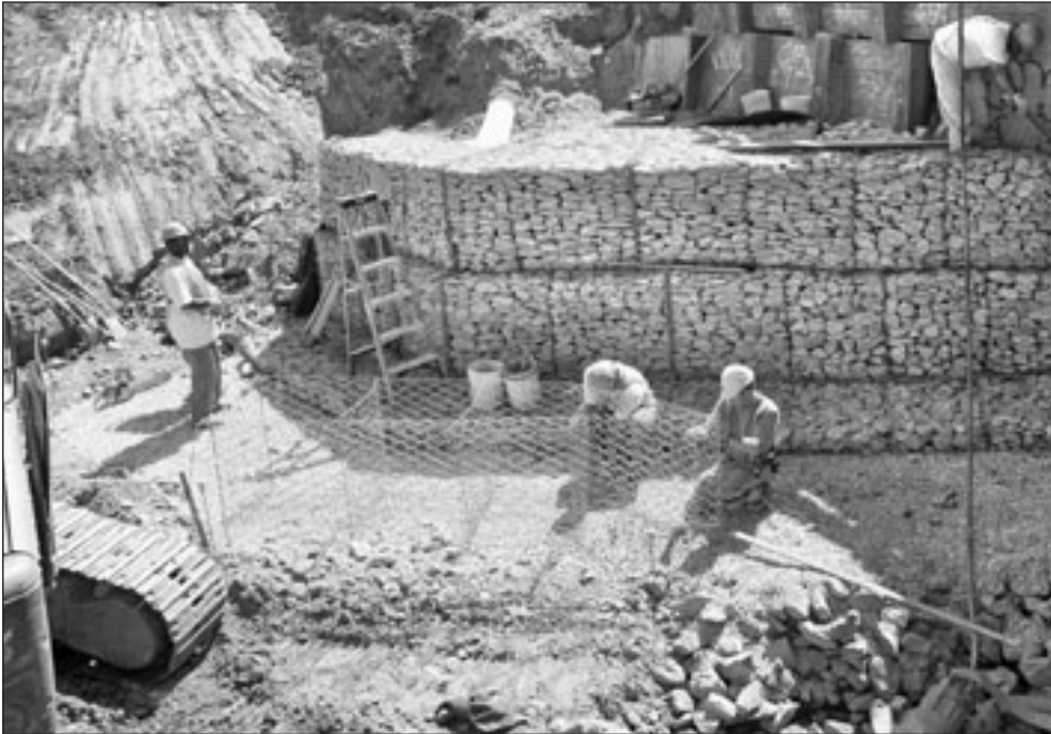
Assembling one of the gabion retaining wall sections for Little Mill Creek
