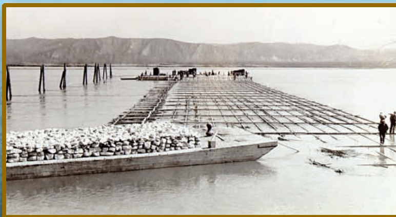
Florence Narrows Dike along the Missouri River in Nebraska at river mile 665.3. This photo was taken in April of 1934. Photo provided
