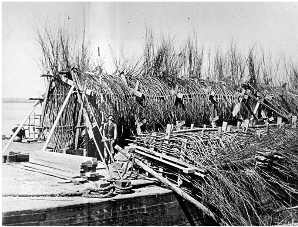
Gabion burs were used historically within streams or rivers for bank stabilization and were placed parallel or diagonal to flows. The gabion burs pictured (below) were built for the Missouri River below Kansas City in 1899. Photo provided
