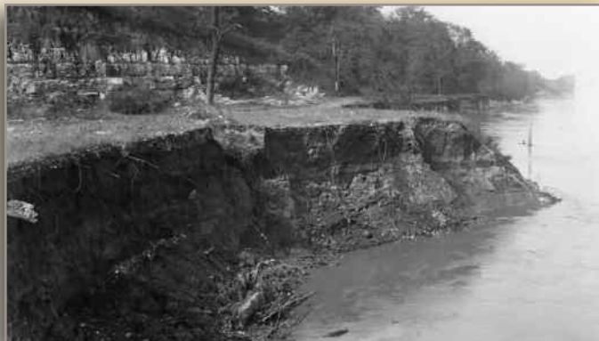
An example of bank erosion
