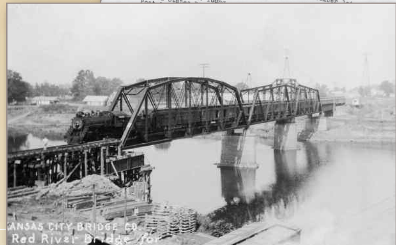
Bridge construction, 1928. Bridge building was another large part of river improvements made by the District
