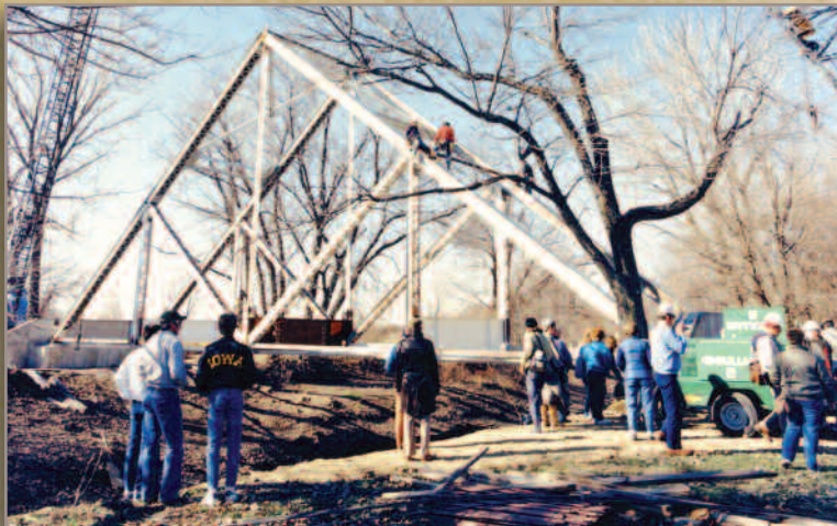
Waddell Truss bridge restoration, 1983. The bridge was moved from Smithville Dam reservoir to Parkville, MO.
