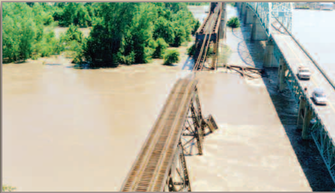
Railroad bridge partly washed out, 1993 flood
