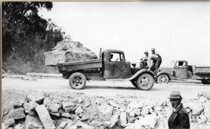
Dam construction workers on the front of the truck are acting as a counterweight for the load of rock in the bed, September 1939
