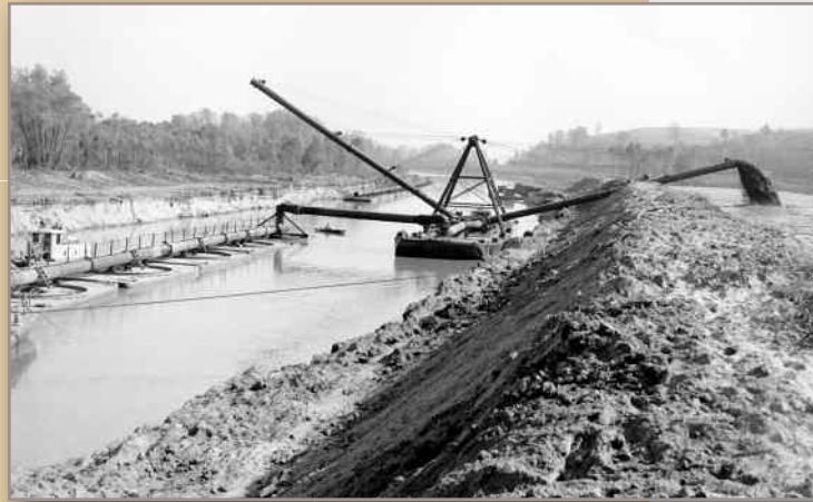
Discharge barge depositing soil behind levee, in connection with the construction of the Liberty Bend cutoff, 1947
