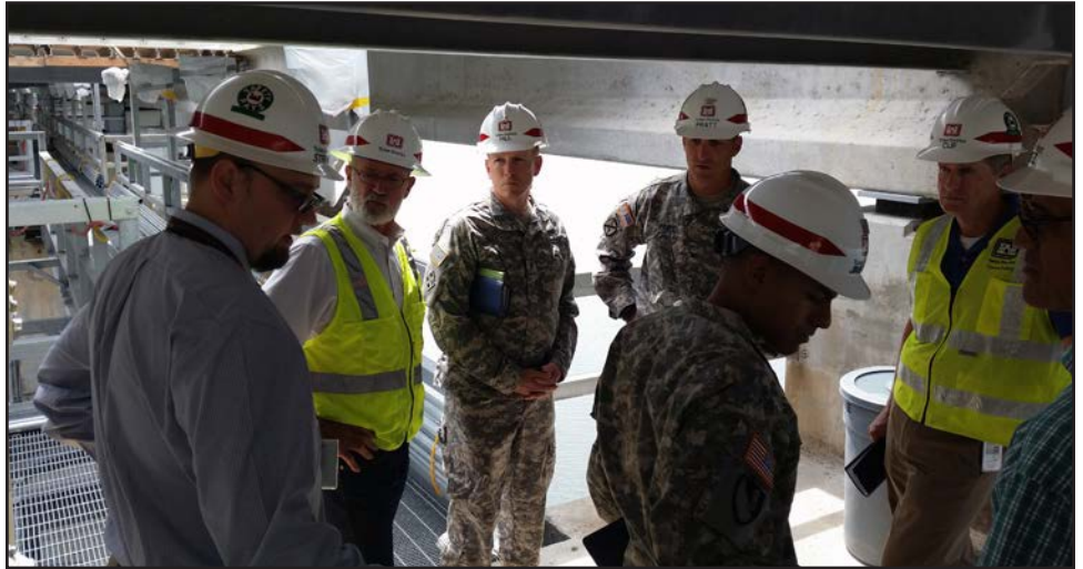
Southwestern Division Commander Brig. Gen. David Hill, Southwestern Division Regional Business Director Pete Perez, and Tulsa District Commander Col. Richard Pratt in the dewatered W.D. Mayo lock chamber August 25. They are standing by the 350,000-pound miter gate, elevated 18 inches by jacks so that the crews can get under it to replace the bushing and pintle ball (the hinge) on which the gate swings. (Photo by Sara Goodeyon)
