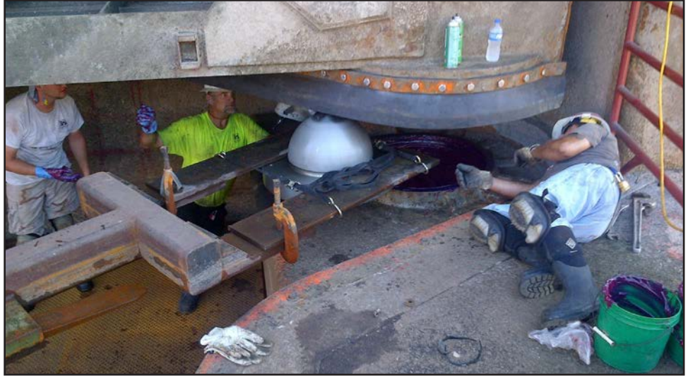
A new pintle ball is moved into place where it will function as a “hinge” for the miter gate at W. D. Mayor Lock and Dam 14. The lock was dewatered, taking just under three weeks for this major maintenance work. (Courtesy photo)
