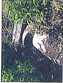
Poorly maintained culvert
