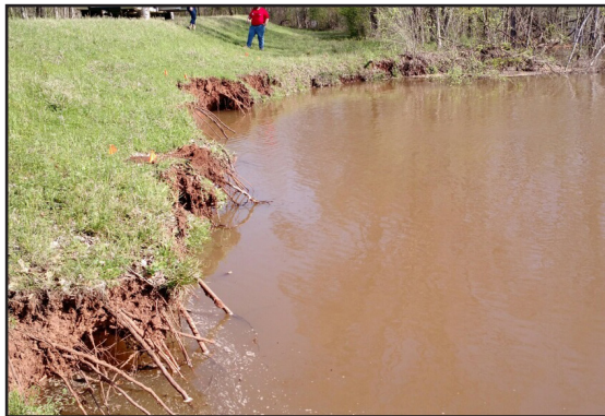
Left photo: Red River Parish, East Point Levee System, compromised by bank caving. (Photo by James McRae)
