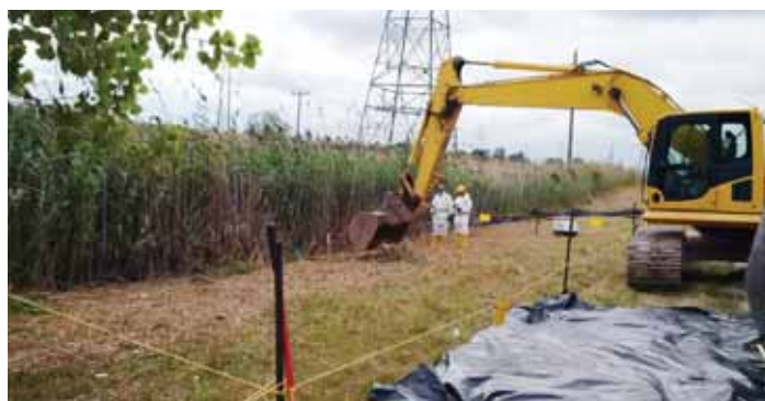
First scoop of soil removed during remediation of the Seaway Site Northside Area
