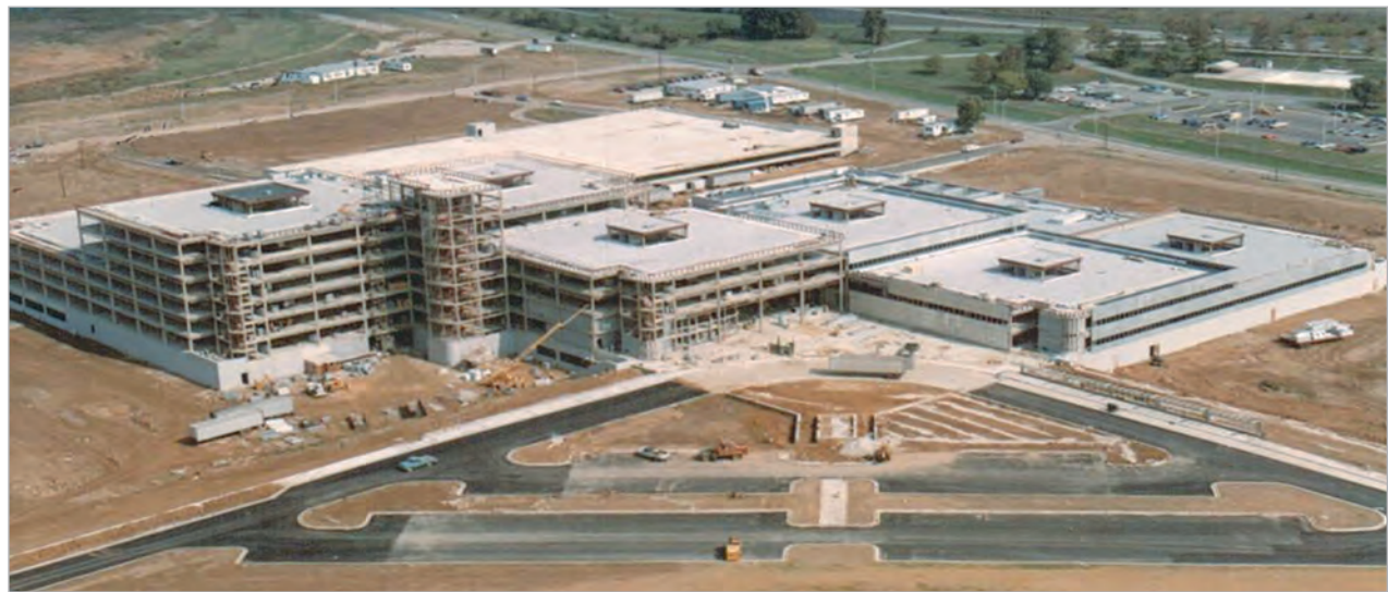
▼ DIA broke ground on the Defense Intelligence Analysis Center (DIAC) in April 1981. By 1982, it was well on its way to completion.
