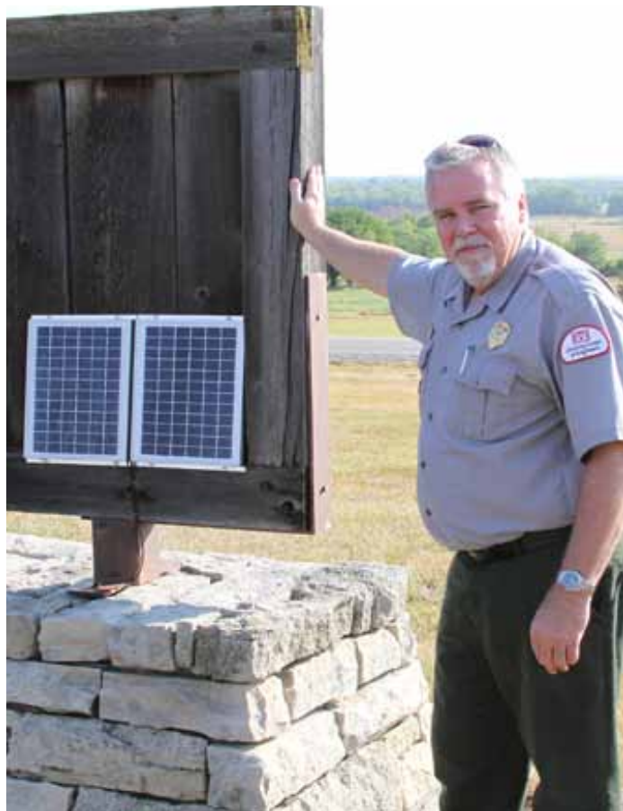
Jim Franz, natural resource manager for Melvern Lake in Melvern, Kan., shows off a solar panel installed to provide energy for LED lights that light the large entrance sign to the lake. Installing solar panel at USACE recreation facilities help USACE cut energy costs. (Photo by Diana McCoy).
