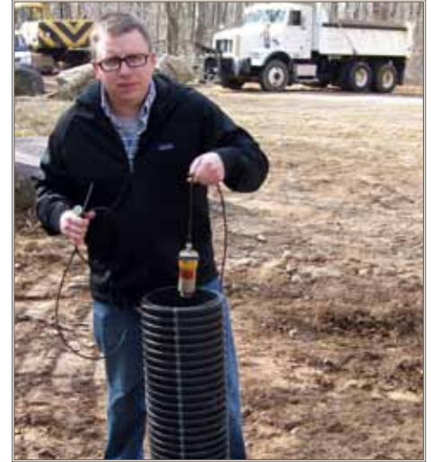
Tobyhanna’s Environmental Management Division personnel install an acoustic leak detection sensor, used to monitor water lines for leaks using sound waves. This innovative approach has applicability across DoD and has been shared across the Army as a best management practice.
