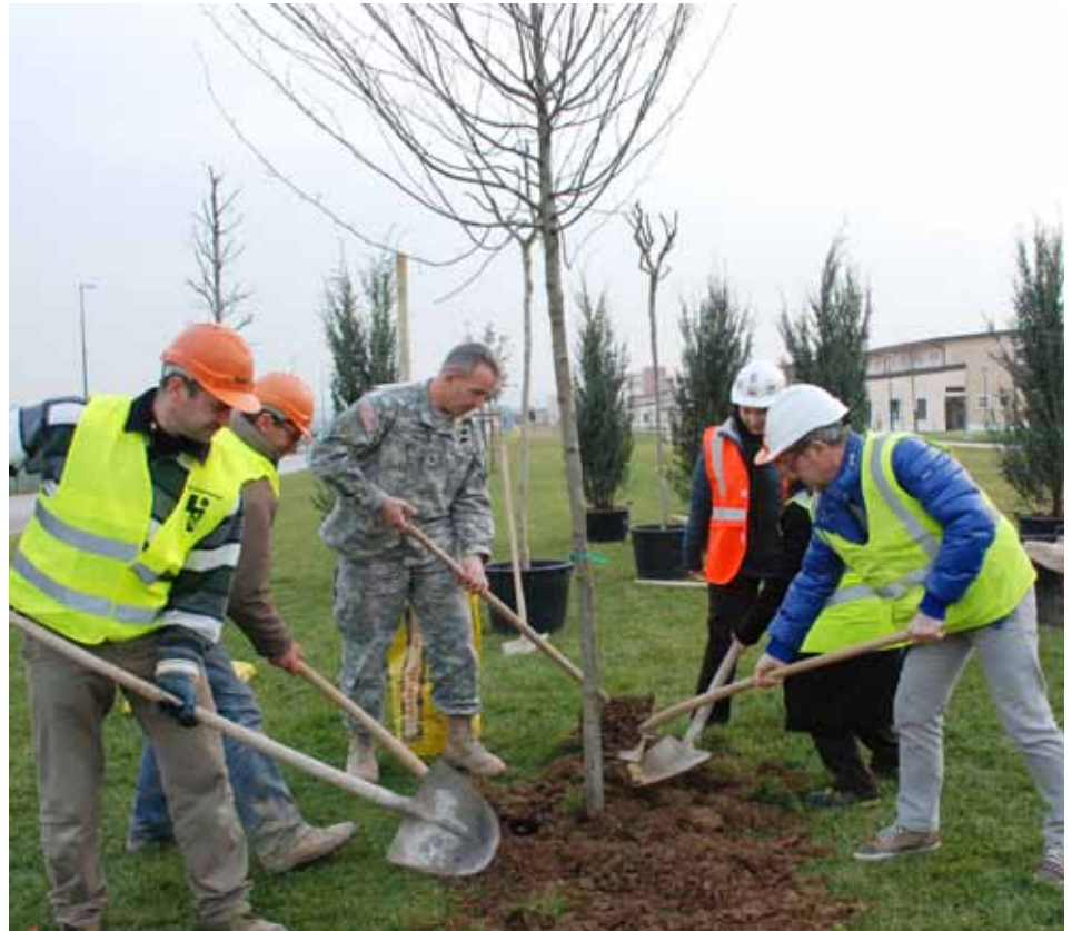
The entire installation covers an area of 145 acres, of which nearly one-third is open green space. This space will also contribute to the LEED Gold rating by implementing water efficient landscaping and use of indigenous plants that thrive on site with minimal care and reduced maintenance cost.
