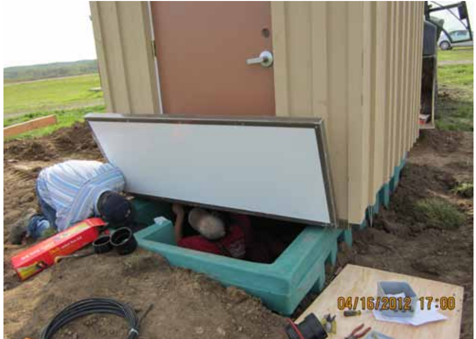
A composting toilet is installed at Camp Atterbury, Ind. between training ranges 18 and 19.
