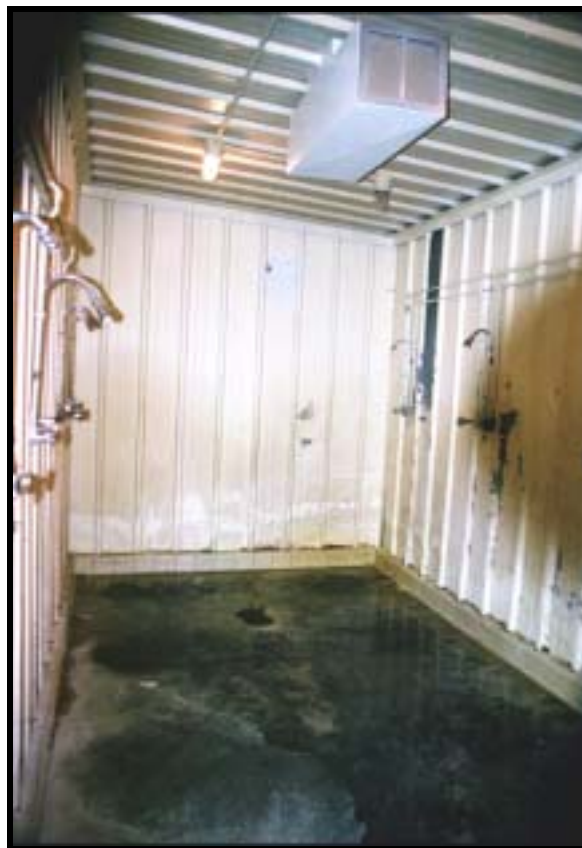
Figure 4.1.227 Showers in mobilization latrine, Bldg. 8128 (1966), Dona Ana Range, Ft. Bliss, view NE (RCG&A).
