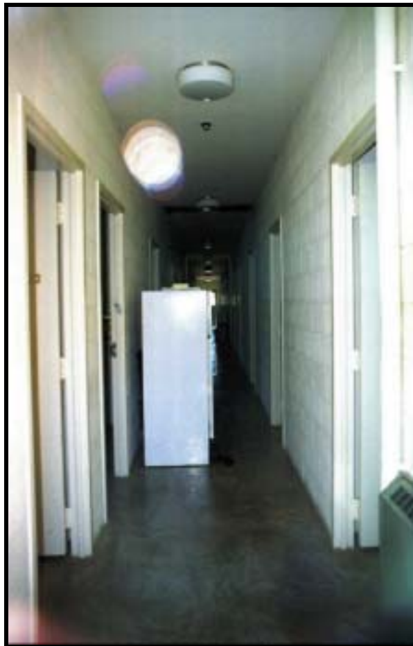
Figure 4.2.56 Army Reserve Annual Training UOQ hallway, Bldg. 56343 (1979), Ft. Hood, view N (RCG&A).
