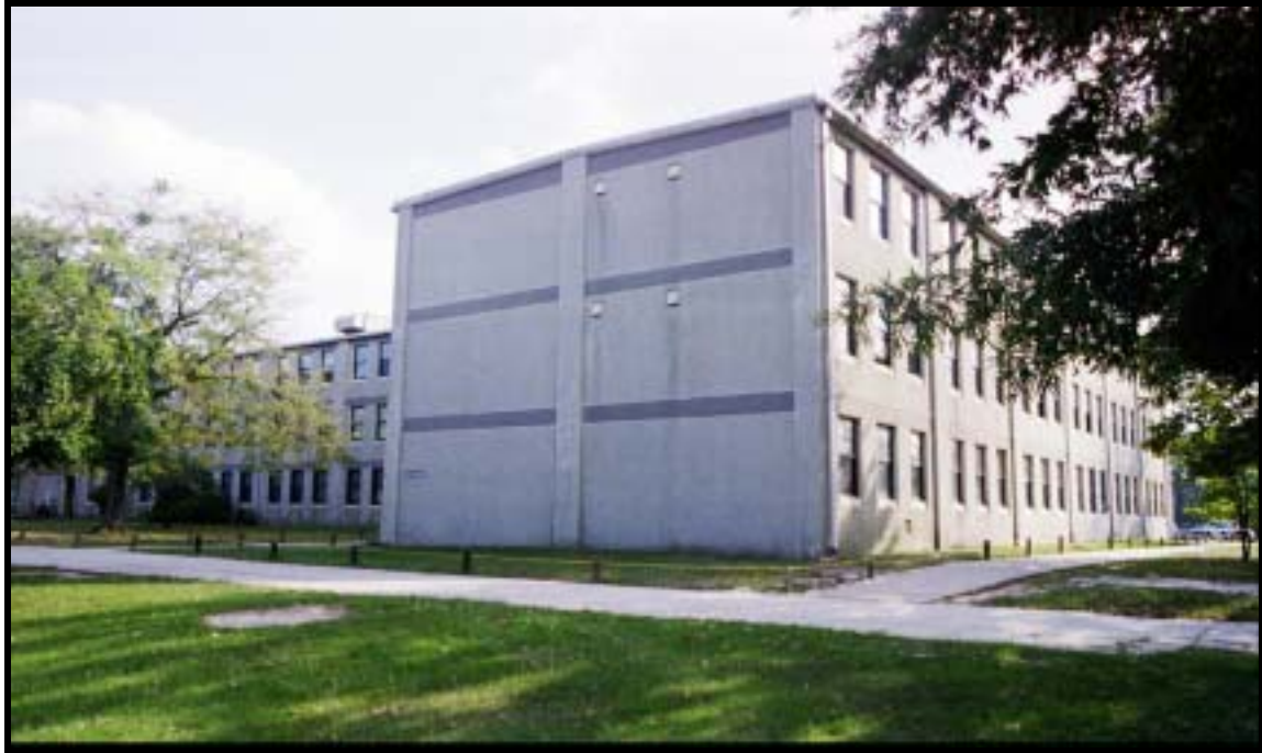
Figure 4.1.59 Alterations to H-style, two-company barracks include new windows and exterior materials, Bldg. C-9349 (1958), Ft. Bragg, view SE (RCG&A).
