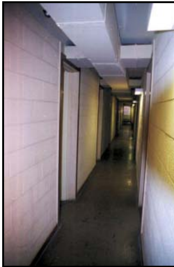
Figure 4.2.82 Semi-permanent “U” BOQ hallway, Bldg. 9517 (1959), McGregor Range, Ft. Bliss, view E (RCG&A).
