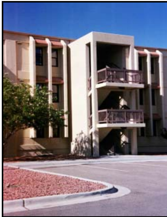
Figure 4.1.34 Detail of exterior renovation to hammerhead barracks, Bldg. 1003 (1956), Ft. Bliss, view NE, (RCG&A).
