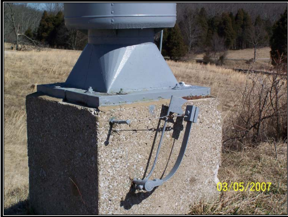
Plate 7.18 Detail of typical igloo ventilator. Note counterweight and flag that would pop-up if ventilator closed (Courtesy U.S. Army, 2007)
