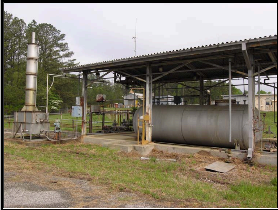
Plate 7.8 Typical storage tank and shelter for inhibited red fuming nitric acid (Courtesy U.S. Army, 2007)
