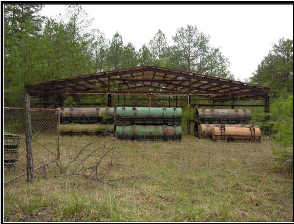
Plate 7.9 Typical outdoor storage area for empty LANCE missile containers (Courtesy U.S. Army, 2007)
