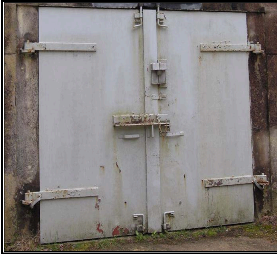
Plate 6.28 Typical igloo door, note ground straps on both lower hinges (Courtesy U.S. Army, 2007)
