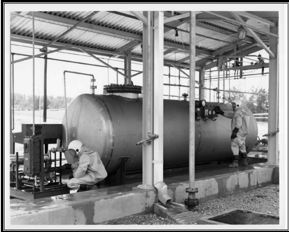
Plate 7.10 Typical fueling operation of liquid-propelled guided missiles ca. 1970. Note full protective gear (Courtesy U.S. Army)
