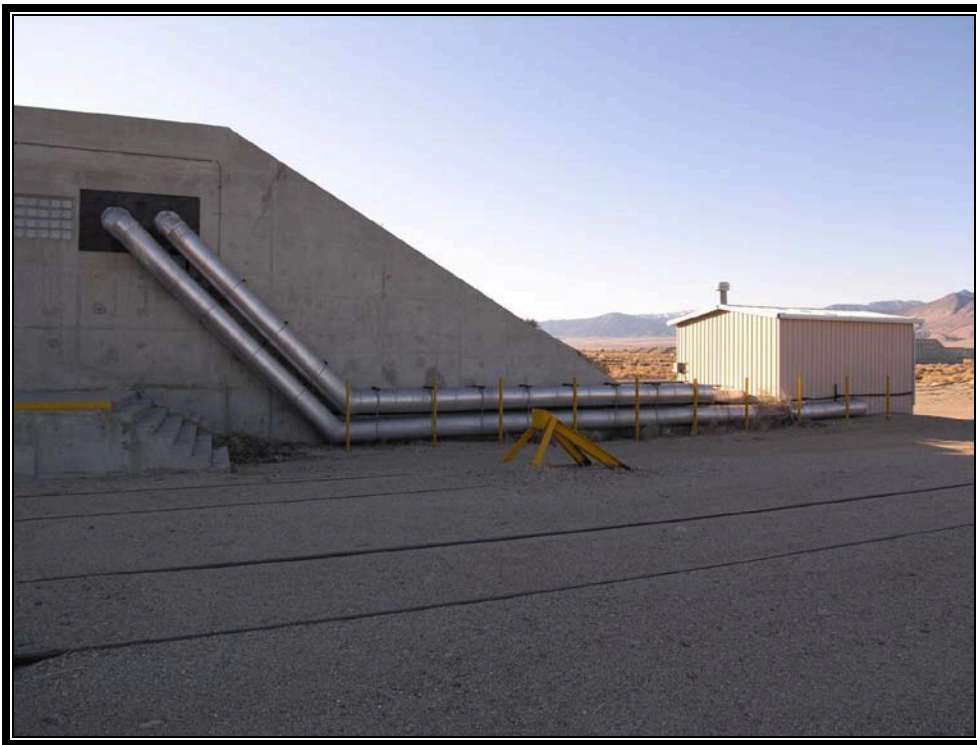
Plate 7.15 Typical earth-covered magazine modified with heating plant to create a constant temperature magazine (Courtesy U.S. Army, 2007)
