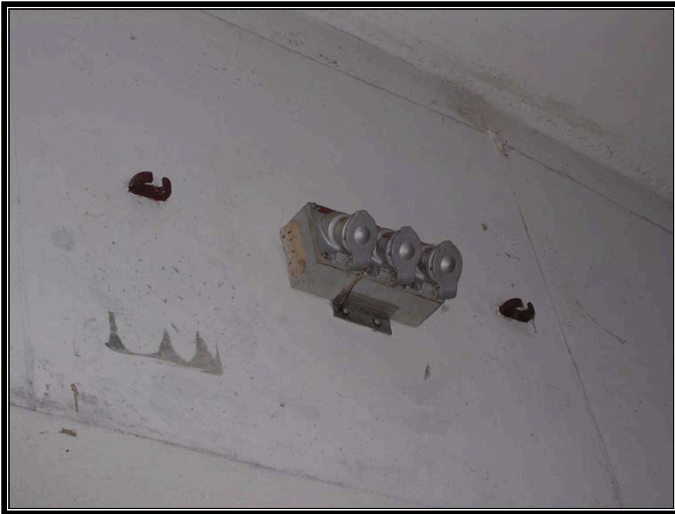
Plate 6.31 Typical explosion-proof electrical connection on interior of igloo. A similar plug on the exterior was connected to a portable generator when electricity was needed inside the magazine (Courtesy U.S. Army, 2007)
