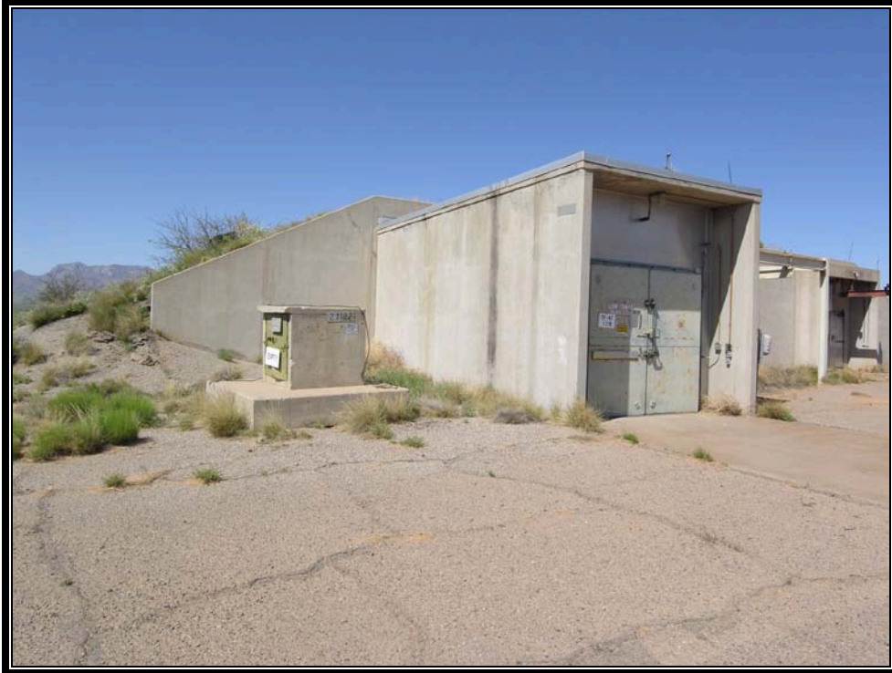
Plate 8.9 The large structure is a climatic test chamber for various munitions. The small structure to the left is a nine square foot magazine (Courtesy U.S. Army, 2007)
