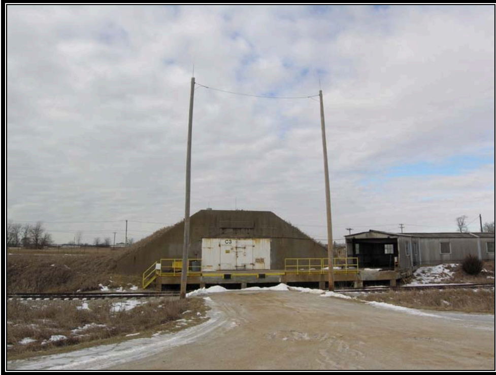
Plate 6.30 Typical shielding system of lightning protection at igloo storage (Courtesy U.S. Army, 2007)
