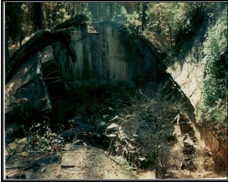
Plate 7.16 Igloo destroyed by detonation of contents, ca. 1955. Note how the force was directed upwards, even though the magazine was totally destroyed (Courtesy U.S. Army)
