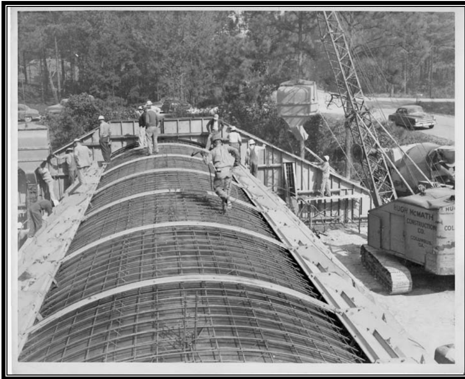
Plate 7.17 Construction of igloo magazines, ca. 1953. Note welder moving across top of arch (Courtesy U.S. Army)
